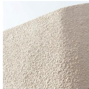
EXTERNAL RENDERED WALL - COLOUR WF-01 PAINTED LIGHT OR SIMILAR TBC BY CLIENT
