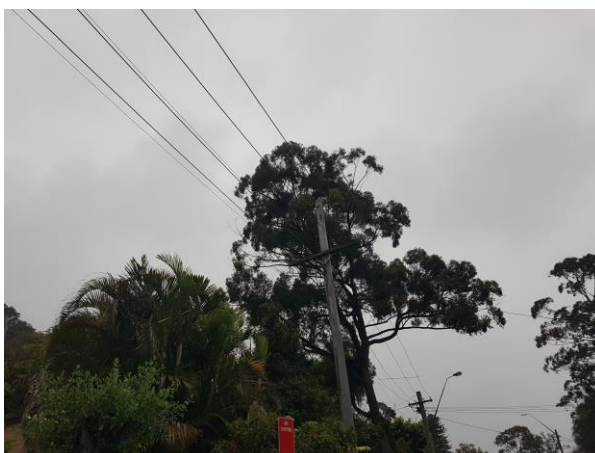
Above ground electrical supply
