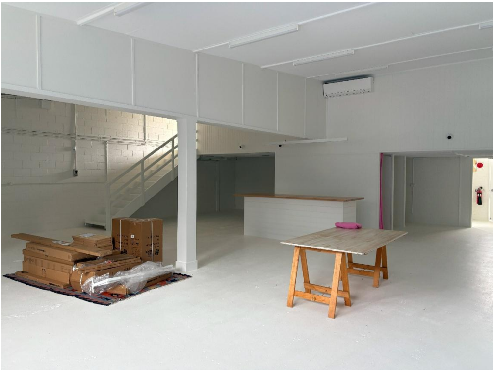
Photograph of the wall removed between Units 6 and 7 / 161-163 South Creek Rd, Cromer
