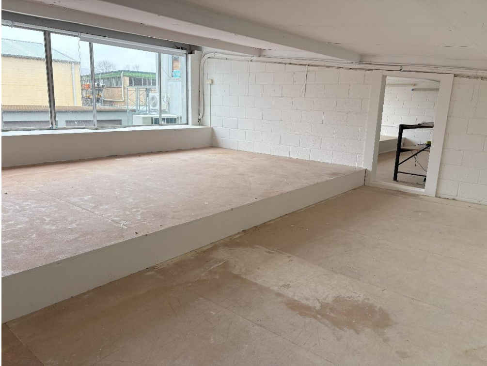
Photograph of the existing mezzanine level with part of wall removed for access between the two areas
