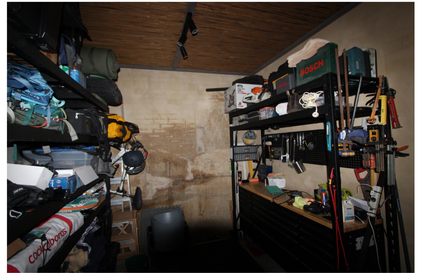
UNAUTHORISED STORE ROOM EXTENSION
