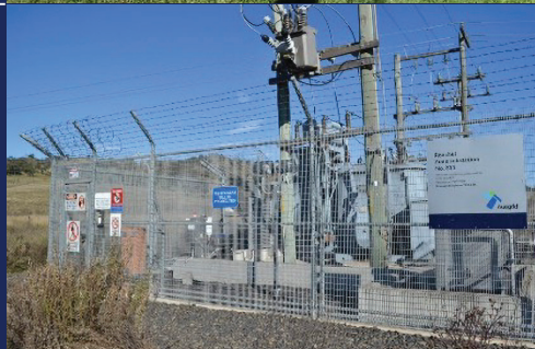
Distribution and Transmission Substations
