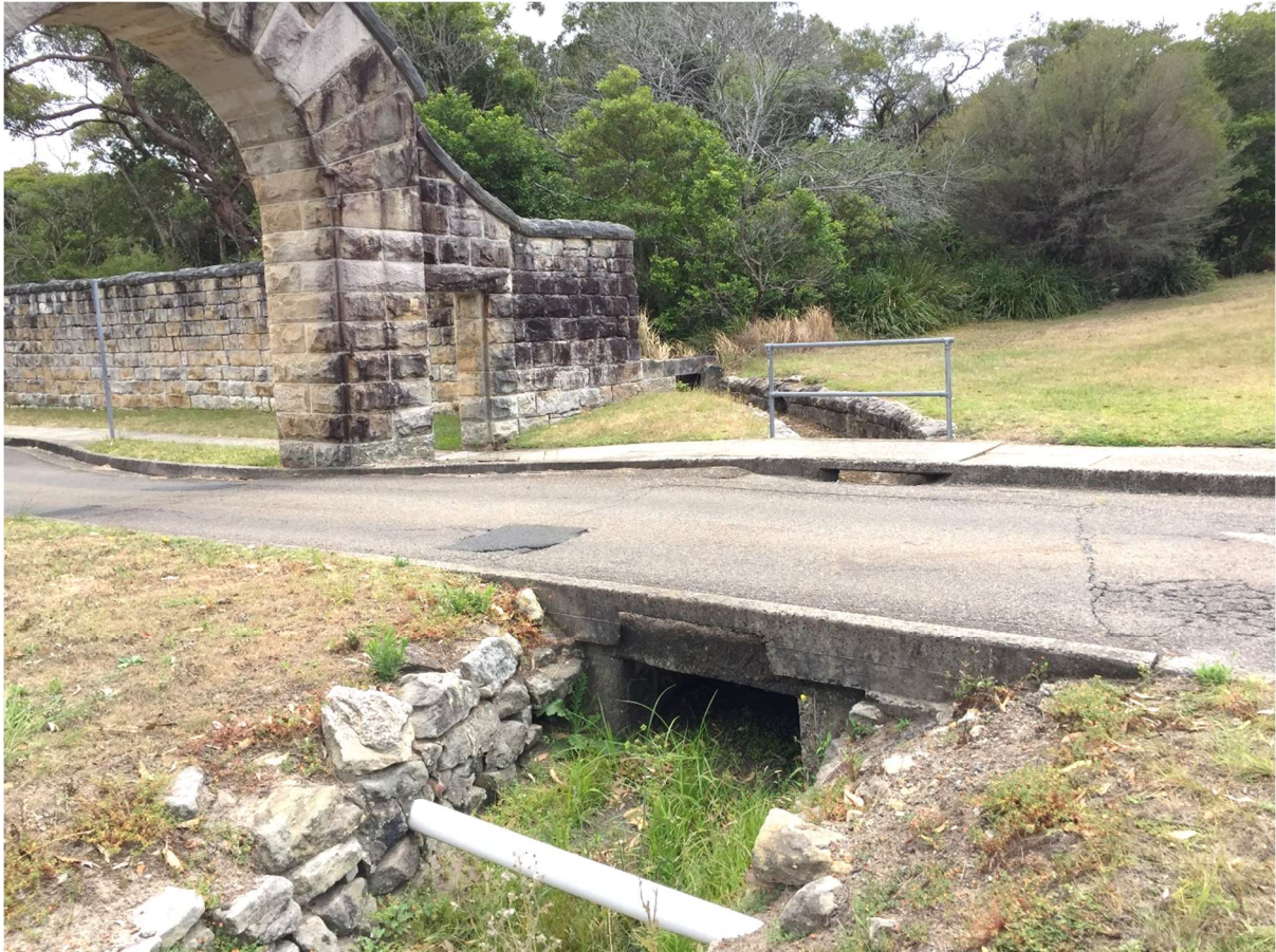
Photo 10: Drainage Channel and Culverts Crossing North Head Scenic Drive
