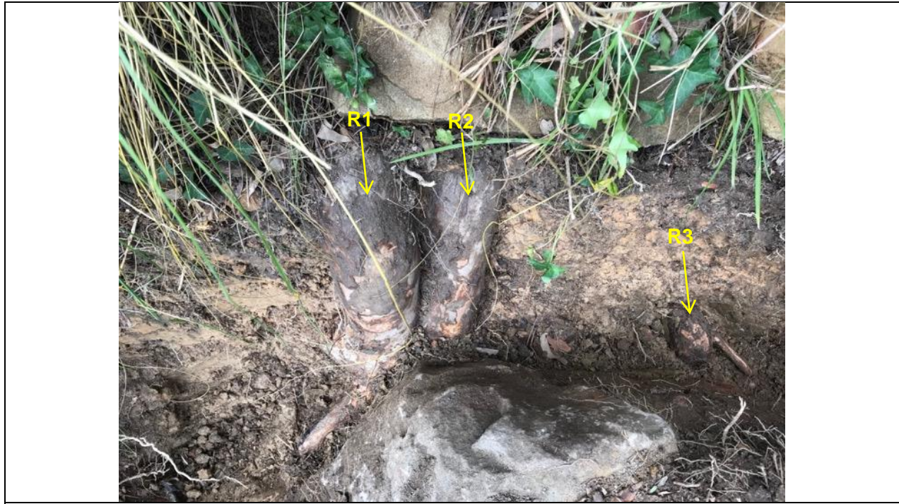
Image 4: Looking South to root investigation trench 1. Showing a close up of root 1, 2 and 3.
