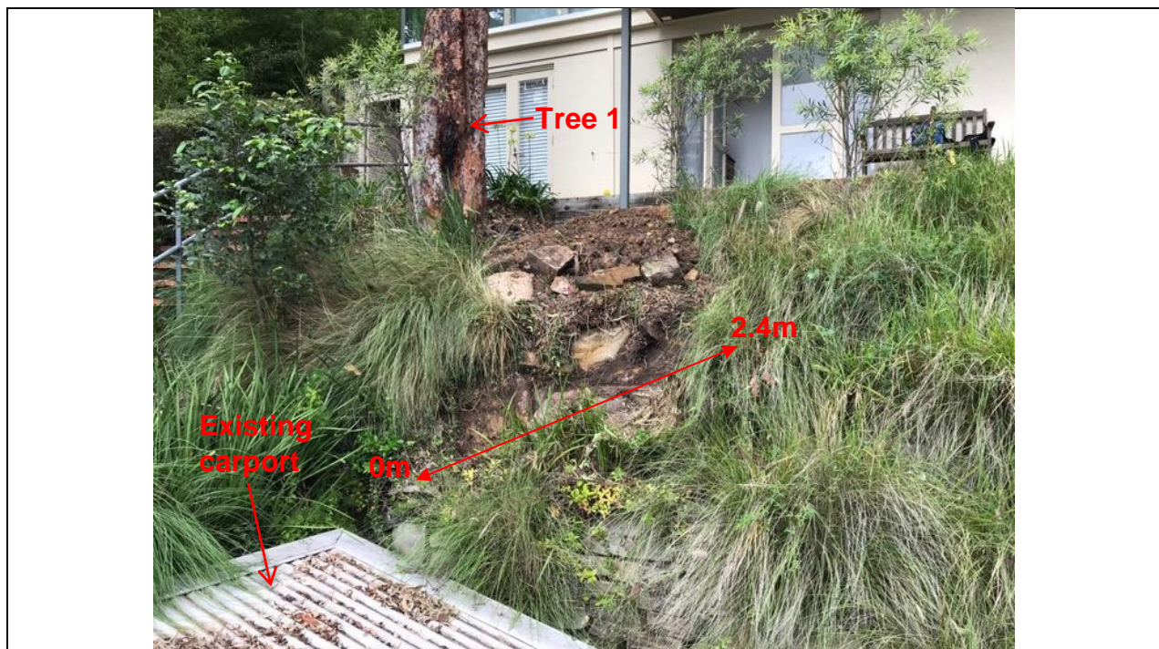
Image 1: Looking South to root investigation trench 1, showing the existing carport, length of trench and tree 1.
