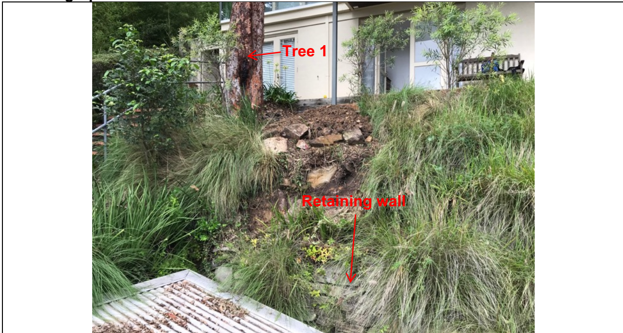
Photo 1: Looking South towards tree 1 from the roof of the existing carport. Showing the existing retaining wall which appears to be restricting root growth into the footprint of the existing carport area.
