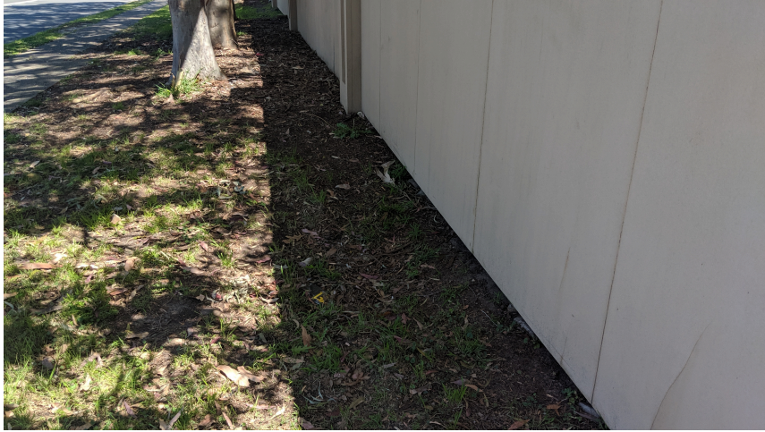
Image 4 - Evidence of scouring along existing wall (South Creek Rd), looking west
