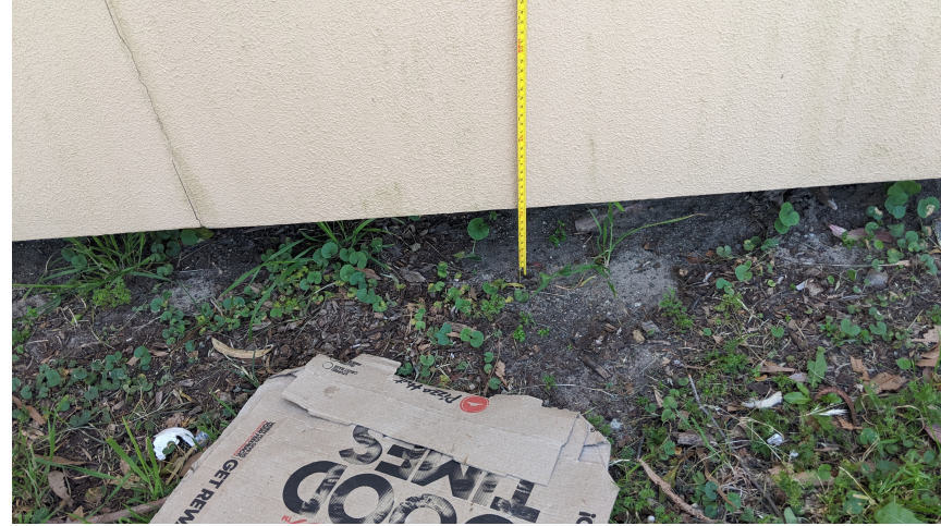
Image 5 - Gap below existing wall (South Creek Rd), evidence of scouring
