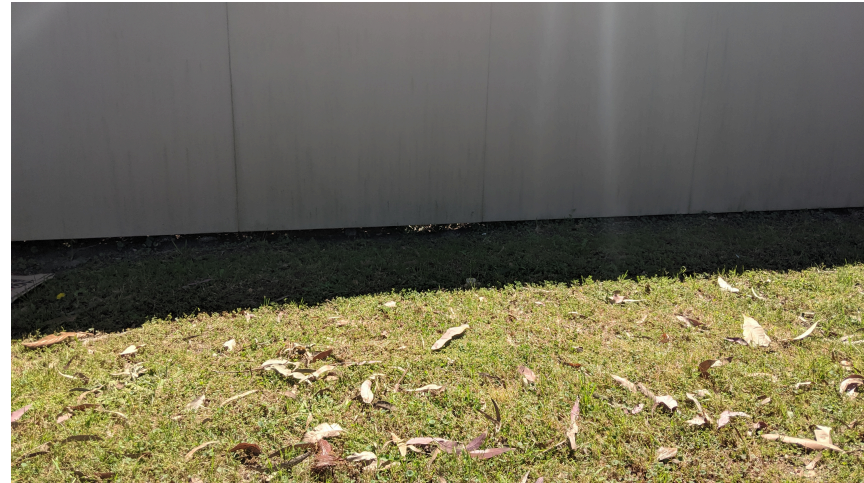
Image 2 - Gaps below existing wall (South Creek Rd)
