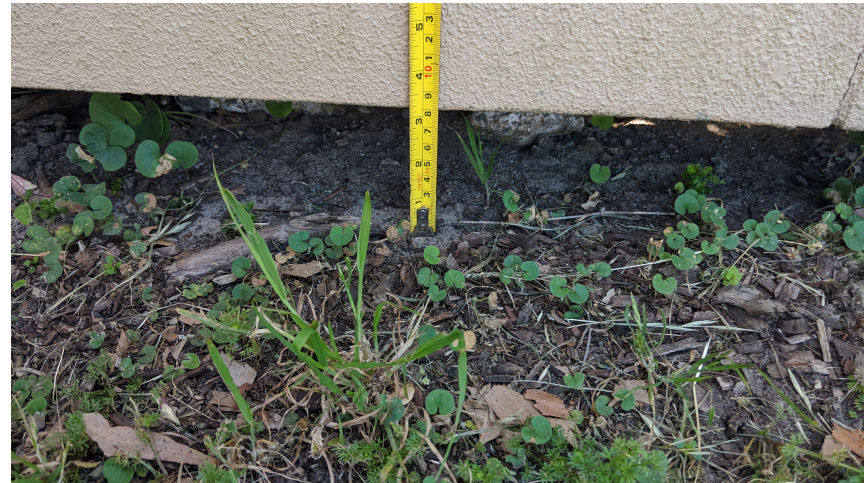
Image 3 - Gap below existing wall (South Creek Rd)
