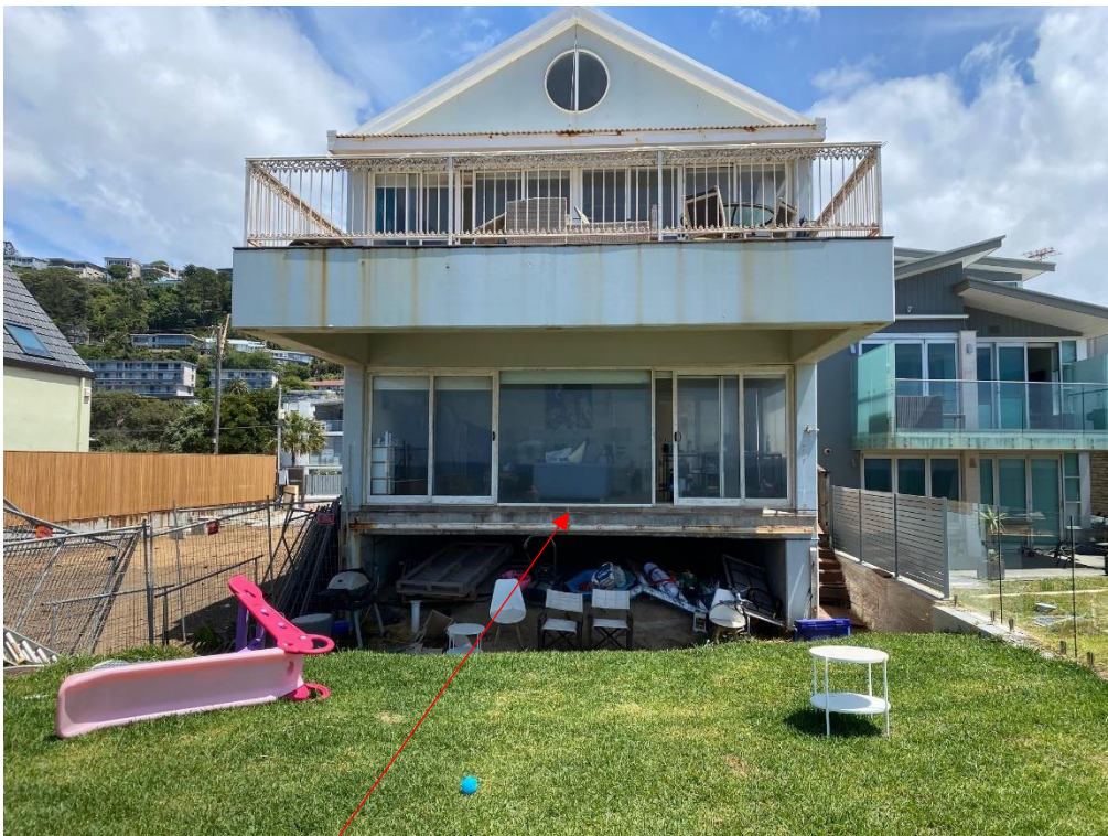
Photograph of rear façade at completion of the sea wall works – noting no ground floor balcony/terrace which was demolished for safety reasons after the 2016 storms
