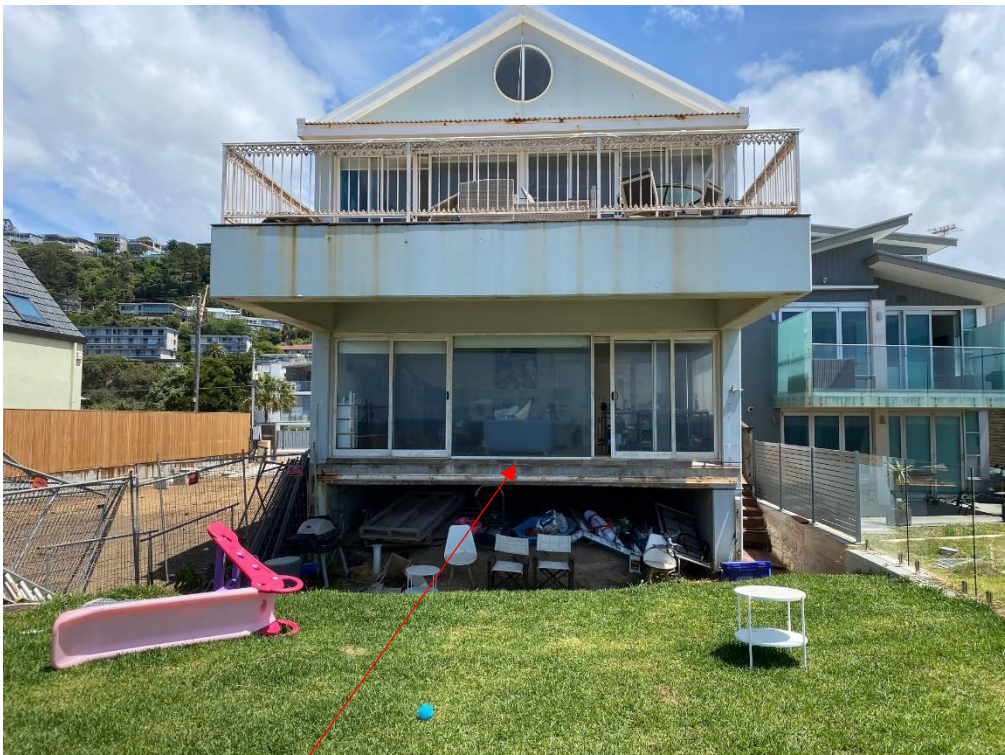
Photograph of rear façade at completion of the sea wall works – noting no ground floor balcony/terrace which was demolished for safety reasons after the 2016 storms
