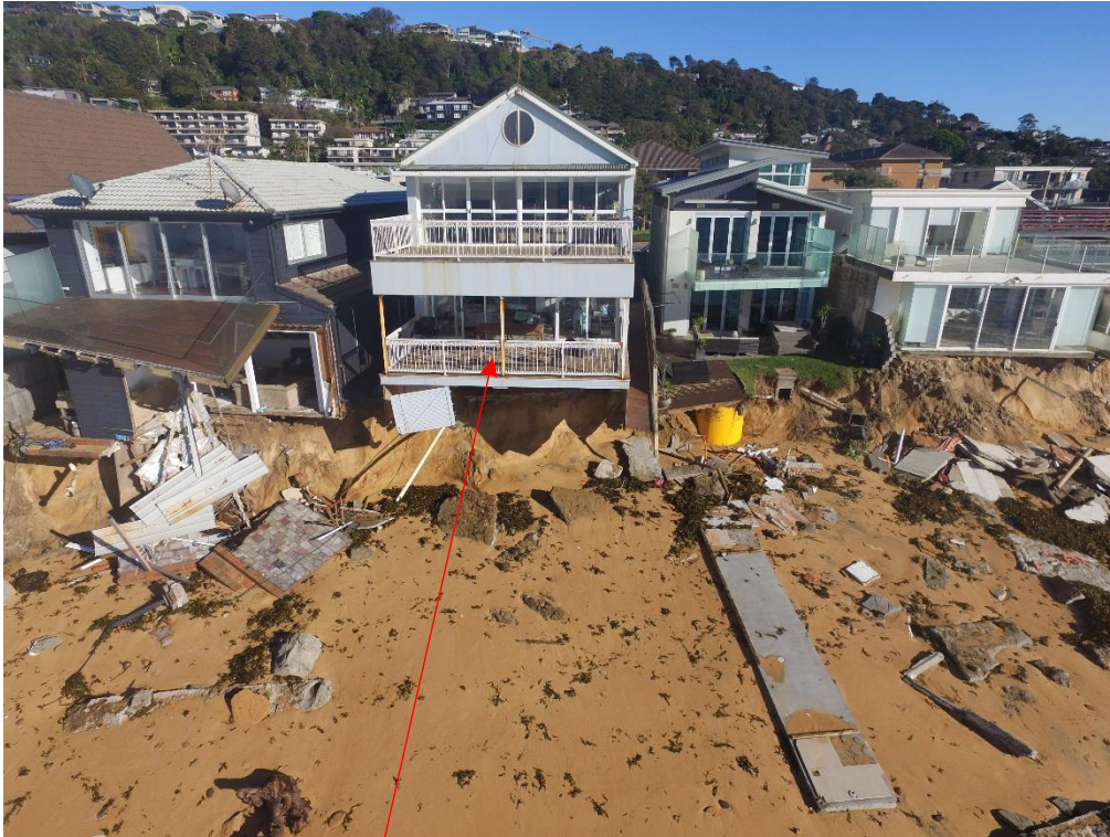
Existing ground floor terrace/balcony and storage at the time of the 2016 Storms prior to being demolished
