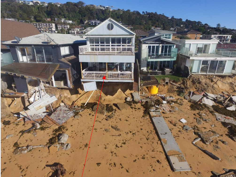
Existing ground floor terrace/balcony with storage under at the time of the 2016 Storms prior to being demolished
