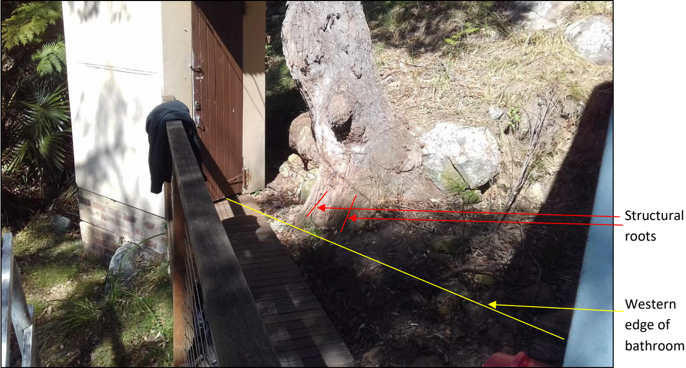
Photo A: Structural roots on the eastern side and recommended western edge of bathroom.
