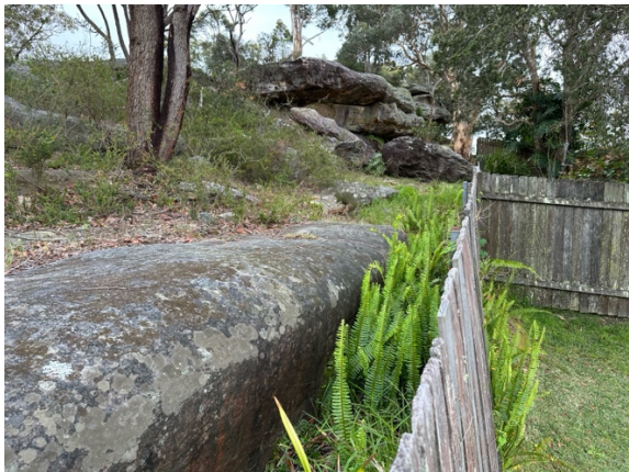
Photo 3: Highly weathered sandstone bedrock outcropping on the rear boundary of the site.
