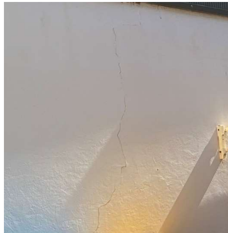
Photograph-10: Cracking within the retaining wall. View looking west.
