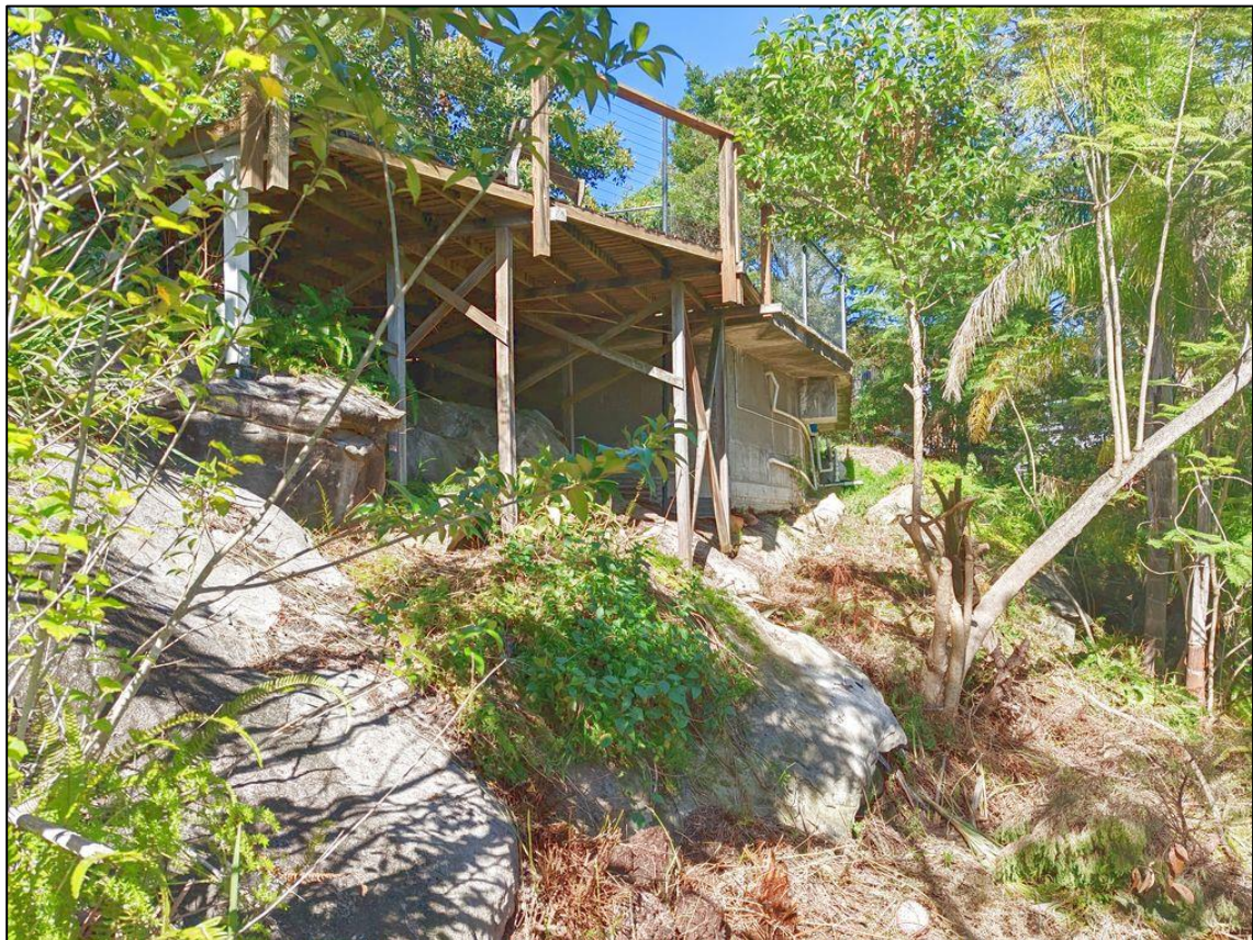
Photograph 6: Showing the area under the pool at 12 Gladys Avenue.
