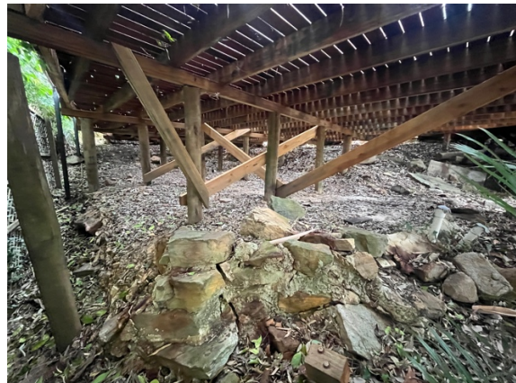
Photo 4: Underside of timber deck in the general area of the proposed works.
