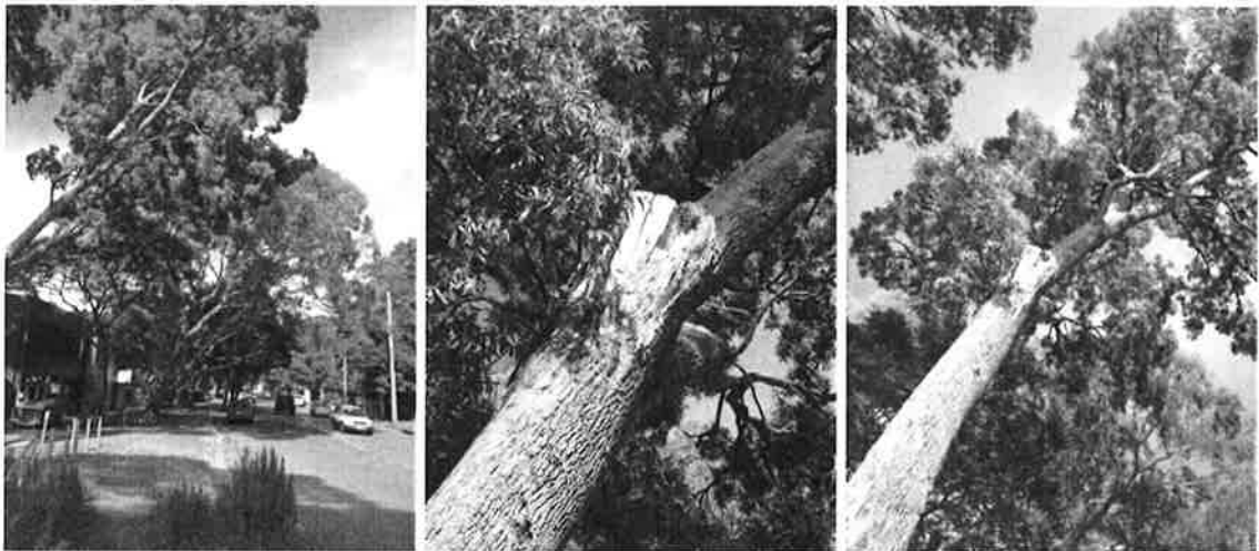
Figure 2, 3 and 4: The overhanging canopy of Tree 1 and the large branch failure wound on the tension side of the trunk.
