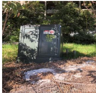
View of the electrical transformer at the north
