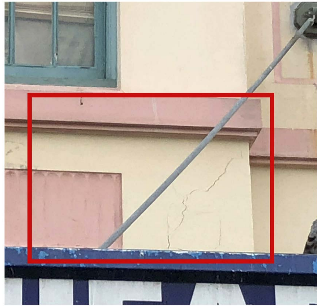
Open-up render and investigate extent of cracking. Rectify cracking to structural engineer and heritage architect's advice and reapply render to match original detail
