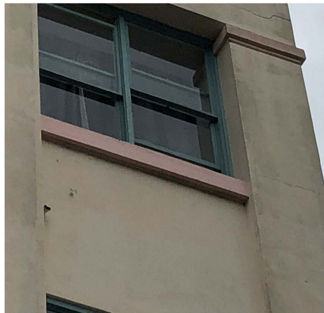
Investigate level of decay of existing windows to determine extent of works. In cases of minor rot, splice in new timbers to replace rotten segments. Where deemed necessary by Heritage Architect, replace windows and frames in timber to match original detail. New glazing shall be provided to all windows to incorporate (20mm max) double glazing units for thermal and acoustic insulation (Thermawood) as directed by heritage architect.
