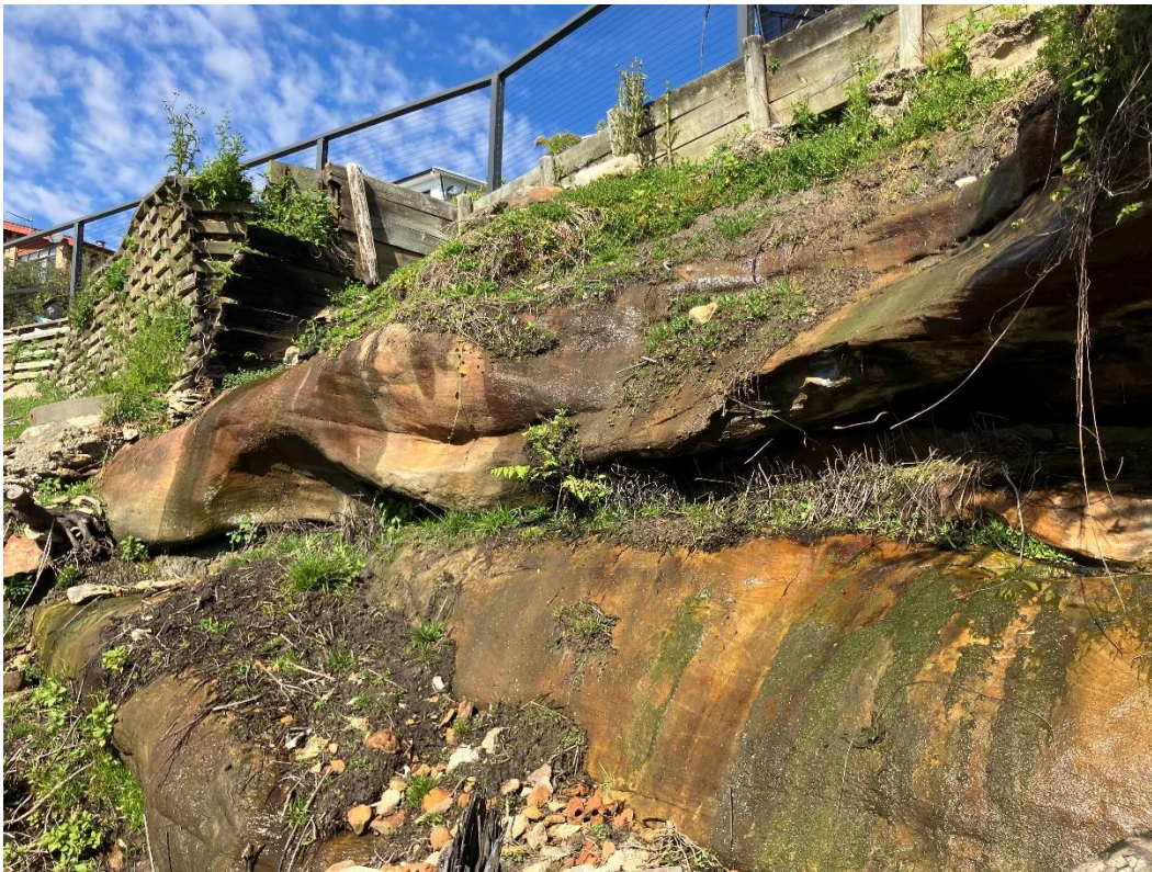
Photograph 3: View of the exposed sandstone bedrock within the rear garden, looking broadly south west, also showing deterioration in the timber retaining wall
