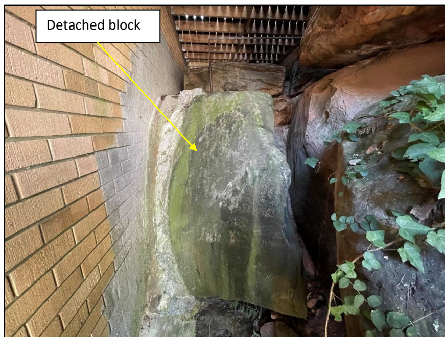
Plate 2: Detached block located against (or possible below) the eastern brick wall of the house
