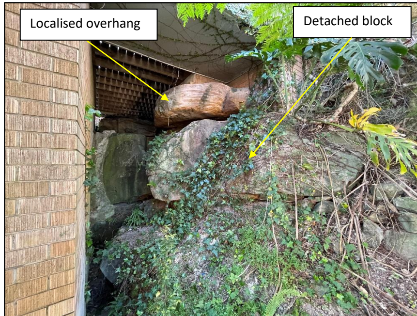
Plate 1: Overhang and detached block located beside the south-eastern corner of the house
