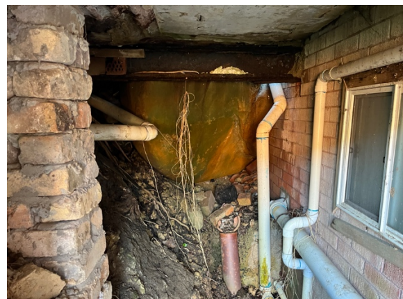
Photo 6: Sandstone boulder under the slab at the south-western corner of the house sits upon uncontrolled fill, sandy materials and brick pieces.
