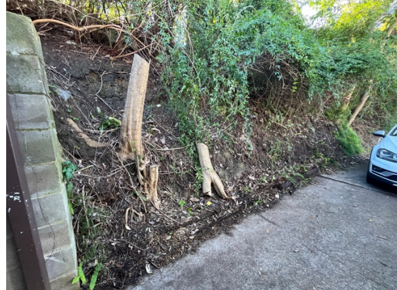
Photo 8: Uncontrolled slope on the western side of the driveway access
