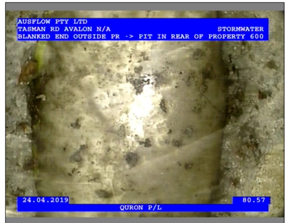
Photo: 3_1_30_24042019_134859_A.JPG 80.57m, Hole in wall , at 12 o'clock
