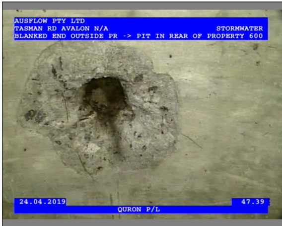
Photo: 3_1_15_24042019_133015_A.JPG 47.39m, Hole in wall , at 12 o'clock
