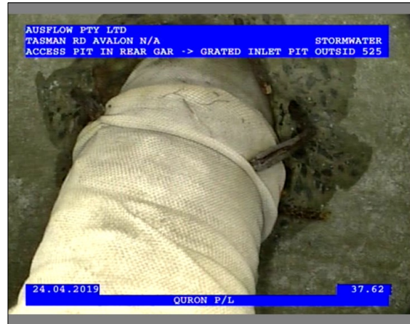
Photo: 2_1_13_24042019_124200_A.JPG 37.62m, Intruding connection, magnitude of intrusion: <5%, General Comments AGGI LINE, at 1 o'clock
