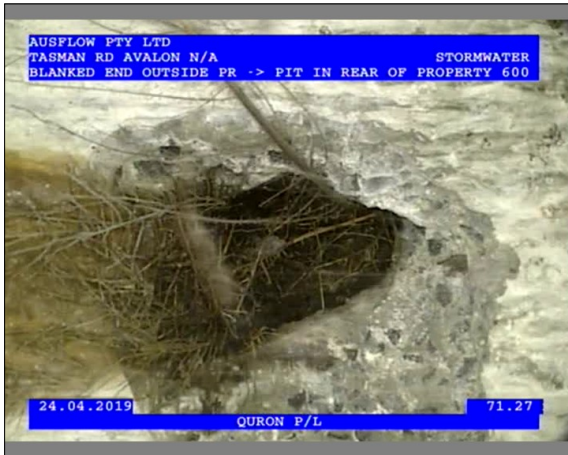
Photo: 3_1_22_24042019_134414_A.JPG 71.27m, Hole in wall , at 9 o'clock
