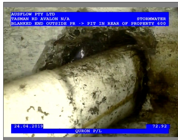
Photo: 3_1_25_24042019_134545_A.JPG 72.92m, Connection, poor workmanship, connection appears to be open , diameter 100mm
