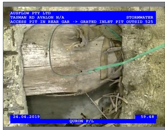
Photo: 2_1_27_24042019_125404_A.JPG 59.48m, Hole in wall , at 12 o'clock
