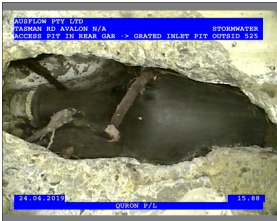
Photo: 2_1_8_24042019_123420_A.JPG 15.88m, Hole in wall , at 3 o'clock
