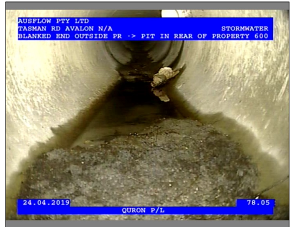
Photo: 3_1_26_24042019_134654_B.JPG 78.04m, Deposit is fine sediments- Sand or Silt in the invert , Obstruction: 5-20% , from 5 to 7 o'clock
