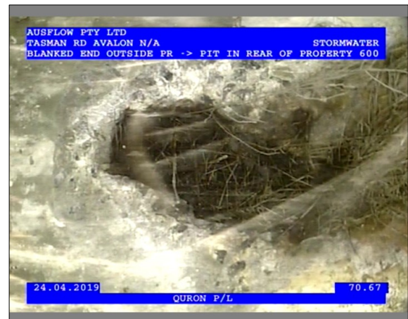
Photo: 3_1_21_24042019_134342_A.JPG 70.67m, Hole in wall , at 3 o'clock
