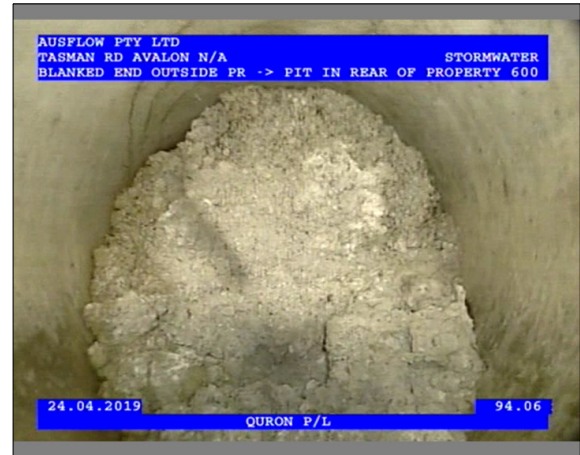
Photo: 3_1_31_01052019_111841_B.jpg 94.56m, Finish node, dead end, Nodename: SPP50849
