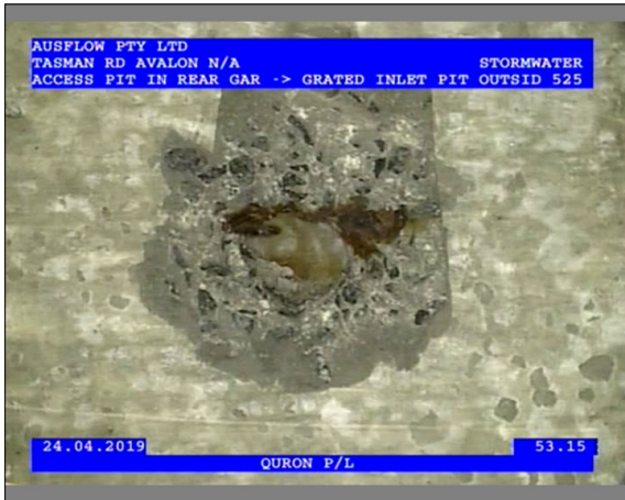
Photo: 2_1_24_24042019_125127_A.JPG 53.15m, Hole in wall , at 12 o'clock
