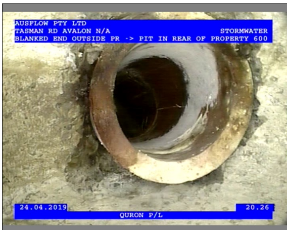
Photo: 3_1_9_24042019_132215_A.JPG 20.26m, Connection, good workmanship, connection appears to be open, diameter 100mm , at 10 o'clock
