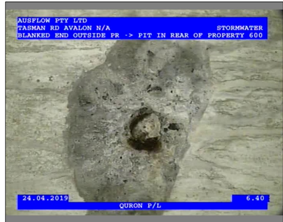
Photo: 3_1_4_24042019_131436_A.JPG 6.4m, Hole in wall , at 12 o'clock
