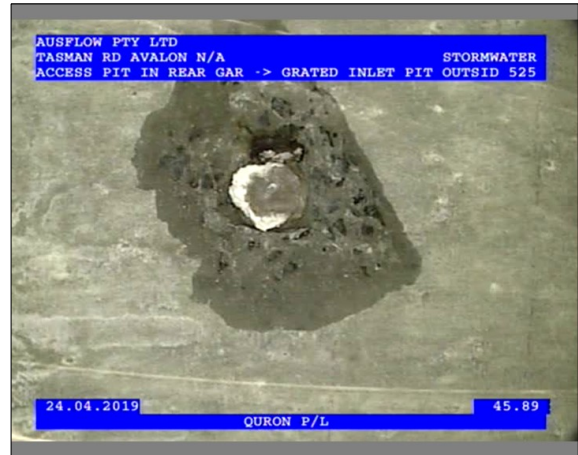
Photo: 2_1_21_24042019_124746_A.JPG 45.89m, Hole in wall , at 12 o'clock
