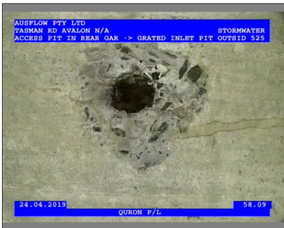
Photo: 2_1_26_24042019_125319_A.JPG 58.09m, Hole in wall , at 12 o'clock
