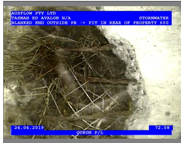
Photo: 3_1_23_24042019_134443_A.JPG 72.08m, Hole in wall , at 9 o'clock
