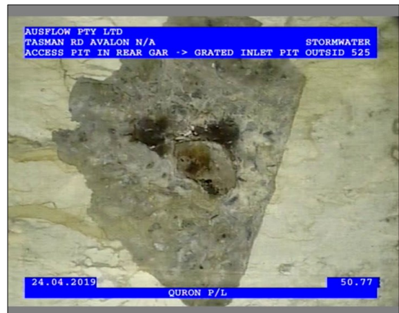
Photo: 2_1_23_24042019_125037_A.JPG 50.77m, Hole in wall , at 12 o'clock
