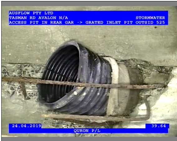
Photo: 2_1_16_24042019_124451_A.JPG 39.64m, Intruding connection, magnitude of intrusion: <5%, General Comments AGGI LINE, at 12 o'clock
