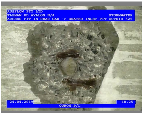
Photo: 2_1_22_24042019_124946_A.JPG 48.25m, Hole in wall , at 12 o'clock
