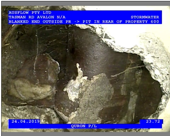
Photo: 3_1_11_24042019_132420_A.JPG 23.72m, Hole in wall , at 9 o'clock
