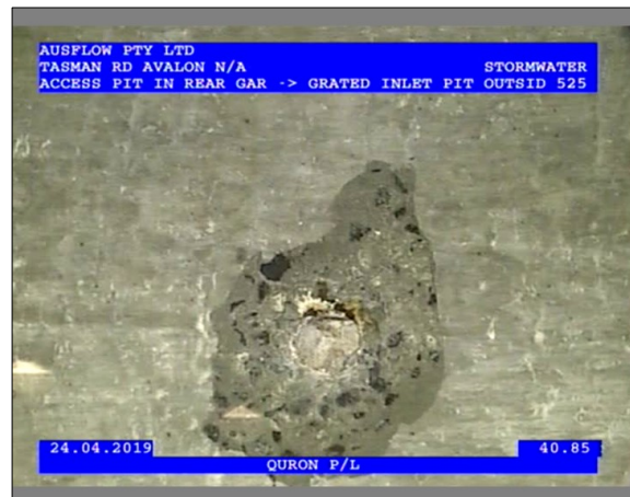
Photo: 2_1_19_24042019_124605_A.JPG 40.85m, Hole in wall , at 12 o'clock
