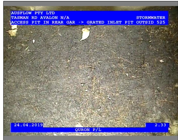
Photo: 2_1_3_24042019_122619_A.JPG 2.33m, Deposit is fine sediments- Sand or Silt in the invert, at joint , Obstruction: 5-20% , from 5 to 7 o'clock
