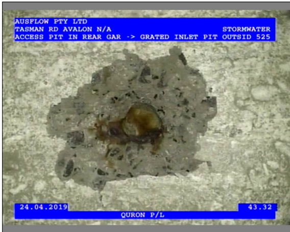
Photo: 2_1_20_24042019_124653_A.JPG 43.32m, Hole in wall , at 12 o'clock
