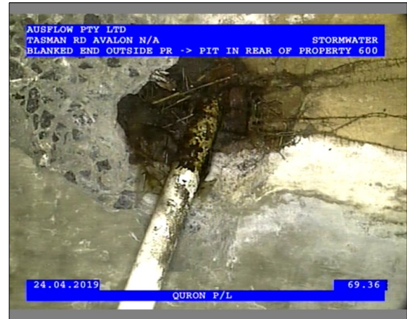
Photo: 3_1_20_24042019_134302_A.JPG 69.36m, Obstruction, an object is intruding through the wall , reduction in cross sectional area: <5%, General Comments CONDUIT, from 10 to 2 o'clock
