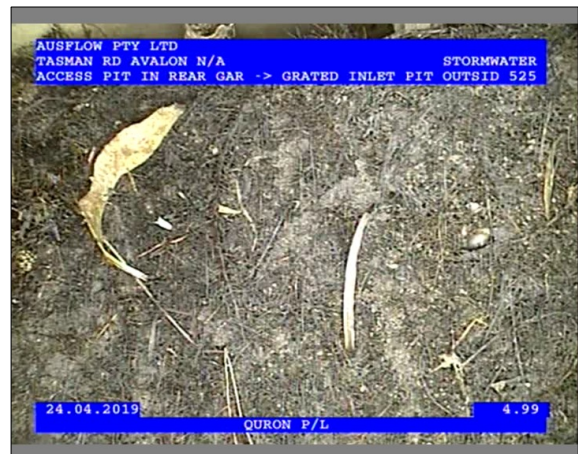
Photo: 2_1_5_24042019_123001_A.JPG 4.99m, A Mass of mostly fine Roots, which has developed into an interwoven clump, at joint, Obstruction: 5-20% , from 4 to 8 o'clock
