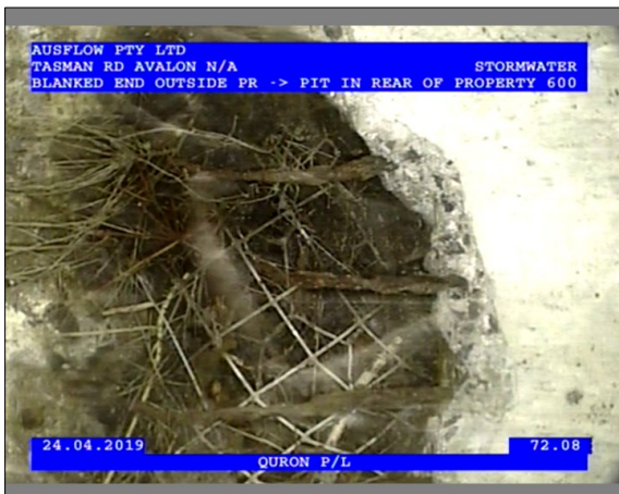
Photo: 3_1_24_24042019_134511_A.JPG 72.08m, Reinforcement is exposed and corroded , at 9 o'clock
