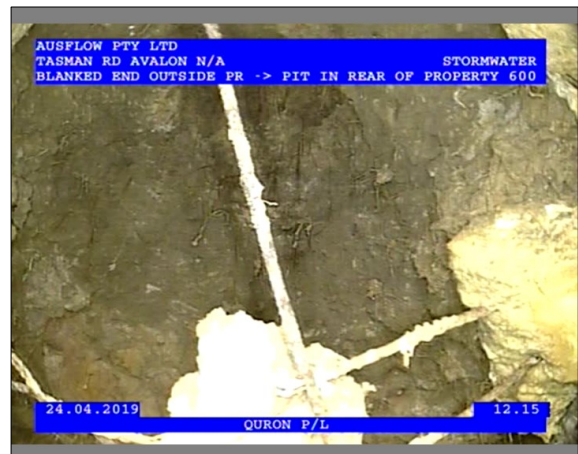
Photo: 3_1_6_24042019_131843_A.JPG 12.16m, Hole in wall , from 11 to 1 o'clock
