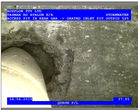
Photo: 2_1_14_24042019_124238_A.JPG 37.95m, Intruding connection, magnitude of intrusion: <5%, General Comments AGGI LINE, at 11 o'clock
