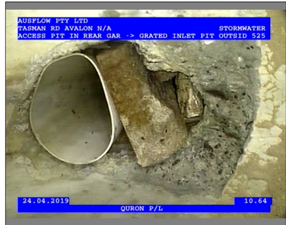
Photo: 2_1_7_24042019_123135_A.JPG 10.64m, Hole in wall , at 9 o'clock
