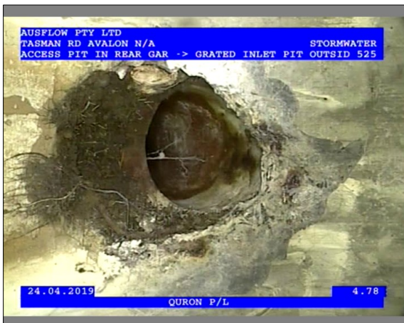
Photo: 2_1_4_24042019_122920_A.JPG 4.78m, Defective Connection - The connecting pipe is damaged, magnitude of obstruction <5%, General Comments NOT FULLY ENTERING PIPE, at 10 o'clock
