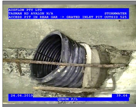
Photo: 2_1_17_24042019_124523_A.JPG 39.64m, Reinforcement is exposed and corroded, at joint , from 10 to 2 o'clock
