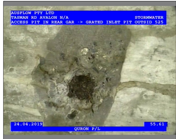
Photo: 2_1_25_24042019_125230_A.JPG 55.61m, Hole in wall , at 12 o'clock
