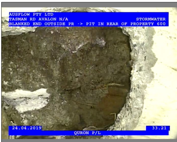
Photo: 3_1_13_24042019_132726_B.JPG 33.21m, Hole in wall , from 9 to 11 o'clock
