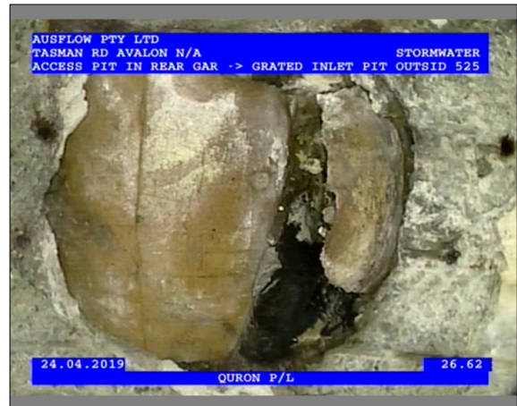
Photo: 2_1_11_24042019_123930_A.JPG 26.62m, Hole in wall , at 2 o'clock
