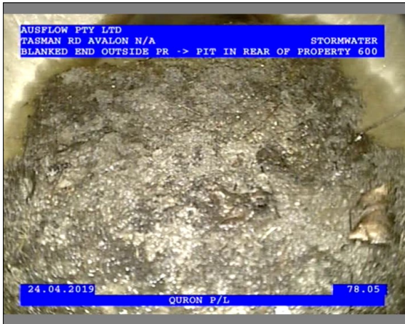
Photo: 3_1_26_24042019_134649_A.JPG 78.04m, Deposit is fine sediments- Sand or Silt in the invert , Obstruction: 5-20% , from 5 to 7 o'clock
