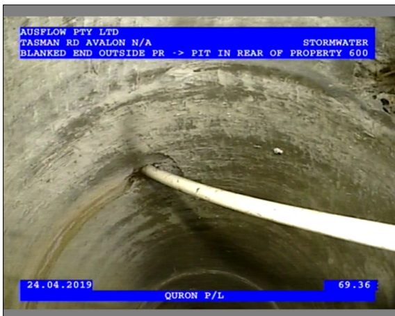
Photo: 3_1_20_24042019_134312_B.JPG 69.36m, Obstruction, an object is intruding through the wall , reduction in cross sectional area: <5%, General Comments CONDUIT, from 10 to 2 o'clock
