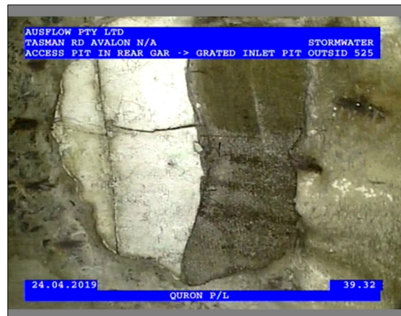
Photo: 2_1_15_24042019_124412_A.JPG 39.32m, Hole in wall , at 3 o'clock
