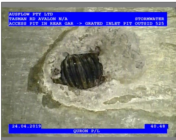
Photo: 2_1_18_24042019_124547_A.JPG 40.48m, Hole in wall , at 1 o'clock
