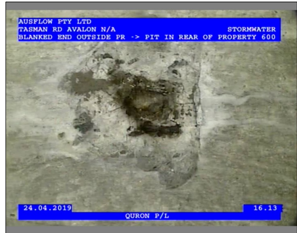
Photo: 3_1_8_24042019_132022_A.JPG 16.13m, Hole in wall , at 12 o'clock
