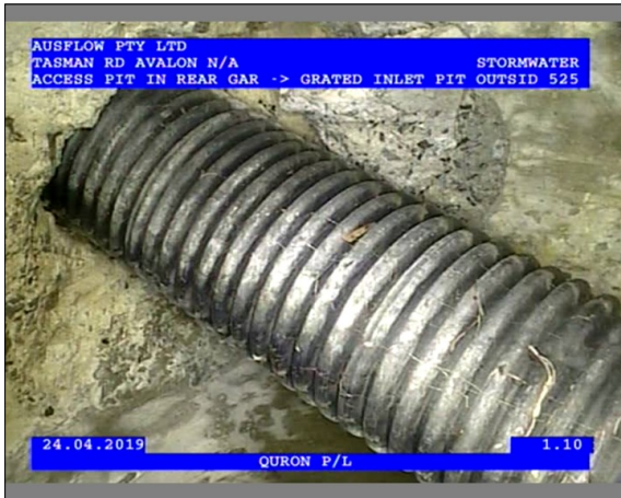
Photo: 2_1_2_24042019_122516_A.JPG 1.1m, Intruding connection, magnitude of intrusion: <5%, General Comments AGGI LINE, at 11 o'clock
