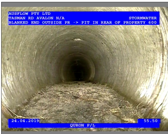
Photo: 3_1_17_24042019_133347_B.JPG 55.5m, A Mass of mostly fine Roots, which has developed into an interwoven clump , Obstruction: 21-50% , from 4 to 8 o'clock
