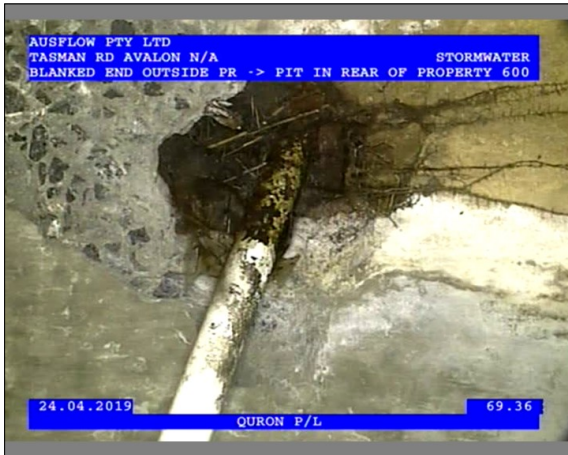
Photo: 3_1_19_24042019_134125_A.JPG 69.36m, Hole in wall , at 2 o'clock
