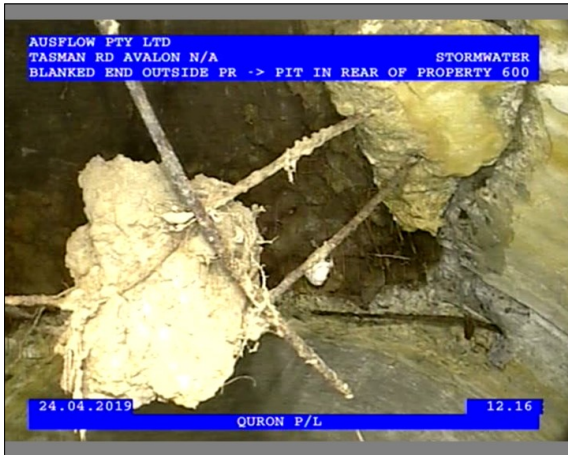
Photo: 3_1_7_24042019_131909_A.JPG 12.16m, Reinforcement is exposed and corroded , from 11 to 1 o'clock
