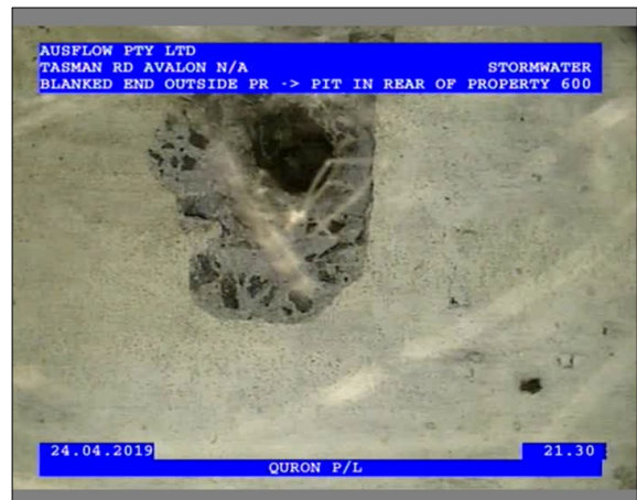
Photo: 3_1_10_24042019_132300_A.JPG 21.3m, Hole in wall , at 12 o'clock
