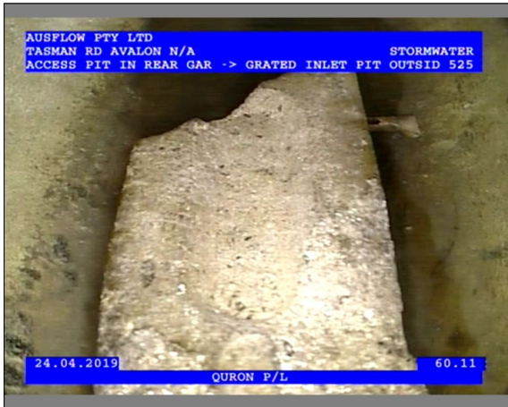
Photo: 2_1_28_24042019_125456_A.JPG 60.11m, Obstruction, dislodged brick or masonry unit lying in the invert , reduction in cross sectional area: 5-20% , at 6 o'clock
