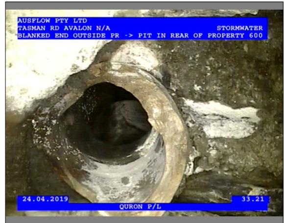
Photo: 3_1_13_24042019_132720_A.JPG 33.21m, Hole in wall , from 9 to 11 o'clock
