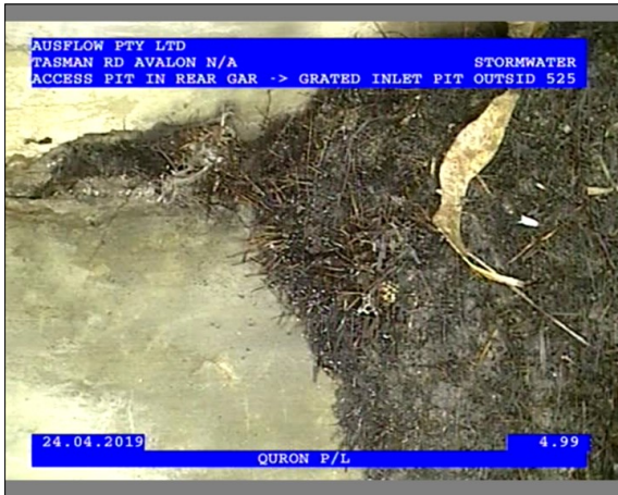
Photo: 2_1_5_24042019_123007_B.JPG 4.99m, A Mass of mostly fine Roots, which has developed into an interwoven clump, at joint, Obstruction: 5-20% , from 4 to 8 o'clock
