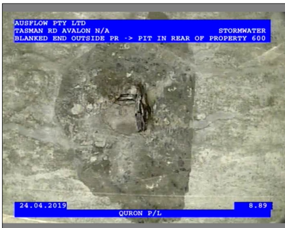
Photo: 3_1_5_24042019_131711_A.JPG 8.89m, Hole in wall , at 12 o'clock
