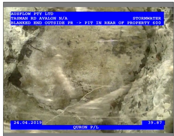
Photo: 3_1_14_24042019_132908_A.JPG 39.87m, Hole in wall , from 10 to 11 o'clock
