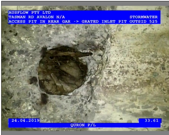
Photo: 2_1_12_24042019_124101_A.JPG 33.61m, Hole in wall , at 3 o'clock
