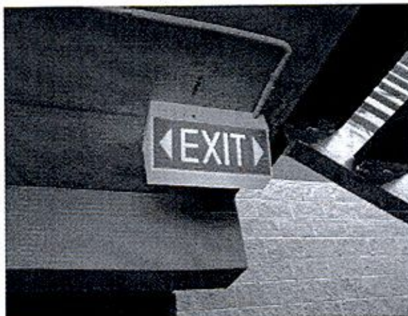
Photo No 8. Exit signs relocated with two arrows added.
