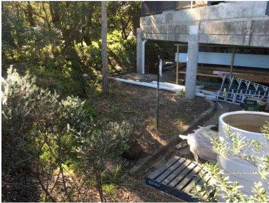
Photo: 1 - Carpark and gutter along west side of down The Newport site
