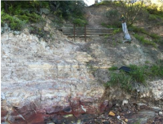
Photo: 3 ó Cliff line at foreshore showing exposed weathered bedrock and erosion along informal pedestrian pathways
