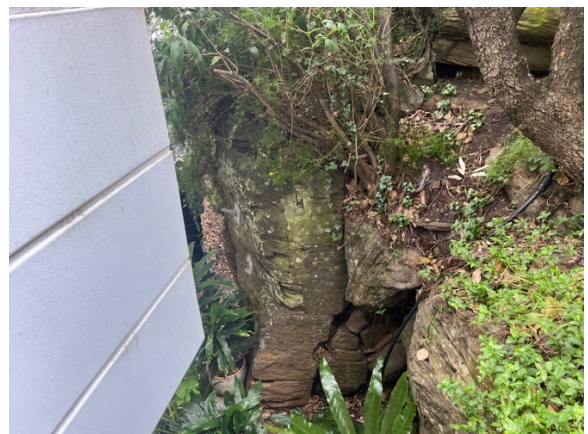
Photo 12: Observed stabilisation works (rock bolts) on the adjoining property. Location is towards the south western corner of the subject site
