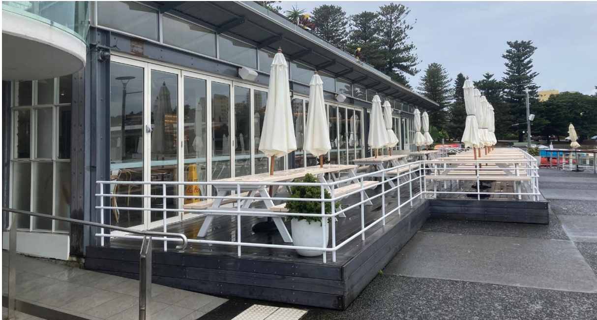
Figure 11: View facing east of existing balustrade at the front of the Manly Wharf Hotel.
