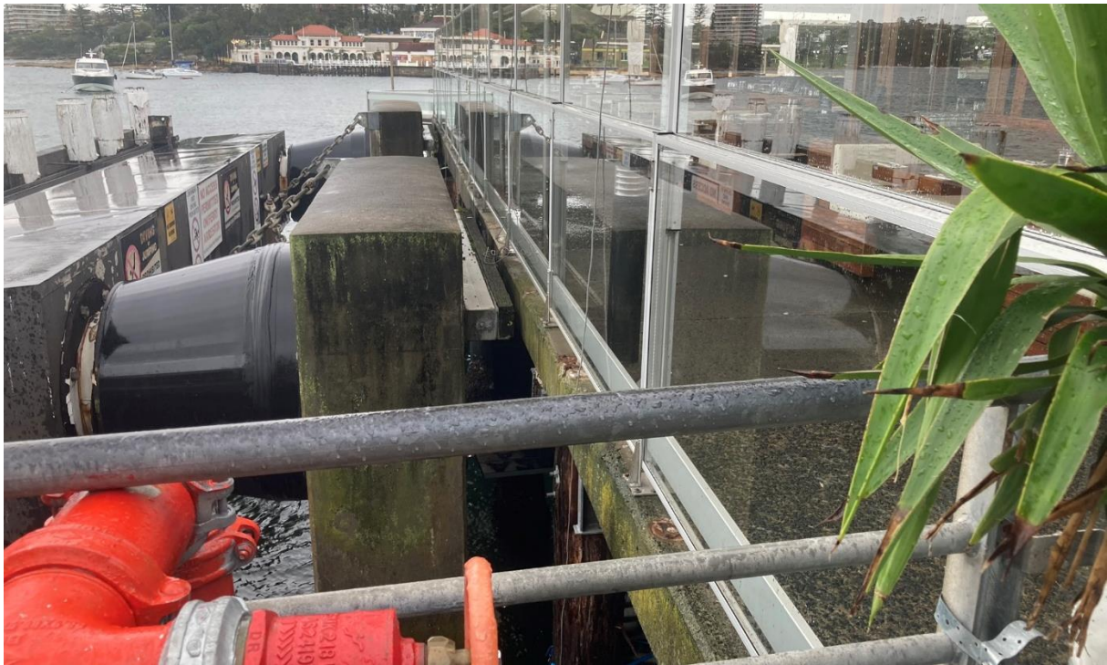
Figure 7: View of an example of the retractable glazed balustrade proposed for the site. This balustrade is outside the Hugos Manly restaurant on the western side of the wharf.
