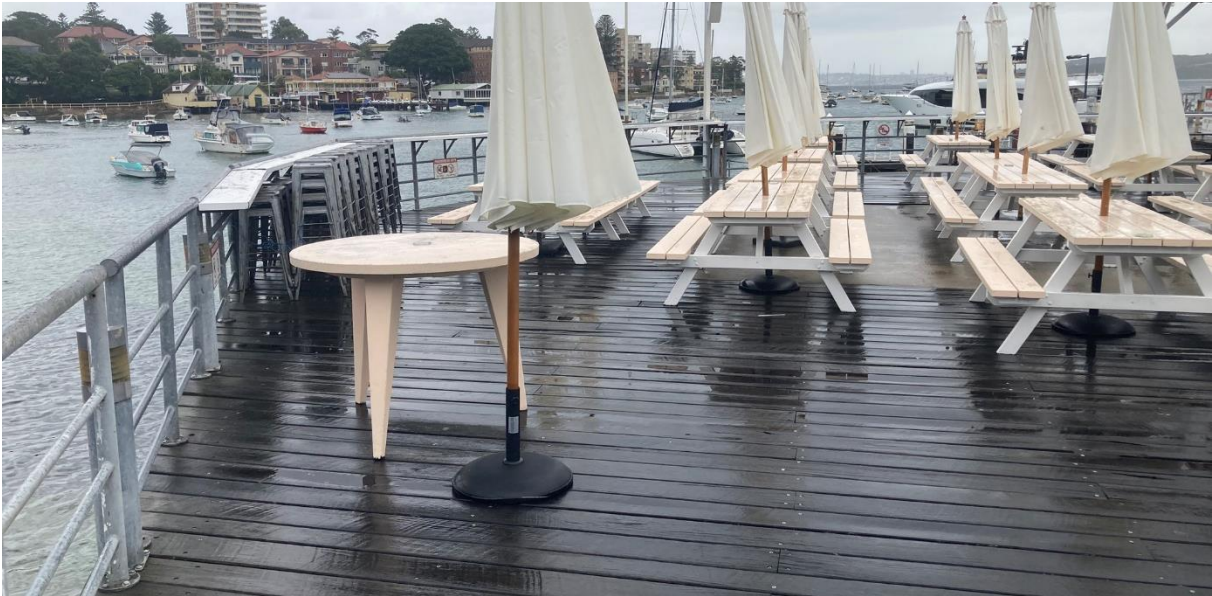
Figure 13: View facing south showing existing balustrade of Manly Wharf Hotel jetty bar to be replaced.
