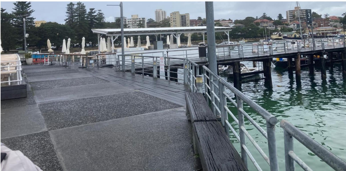
Figure 10: View facing south-east of the existing balustrade along the southern promenade of Manly Wharf.
