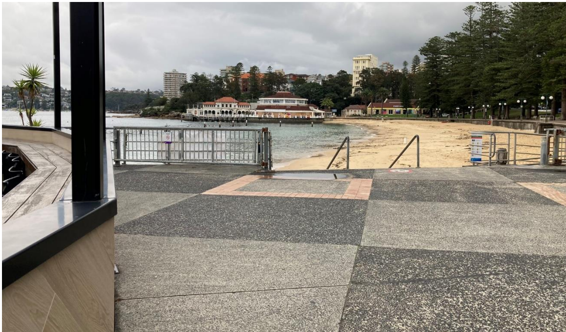
Figure 16: View facing east of existing metal balustrade on eastern side of the wharf to be replaced.
