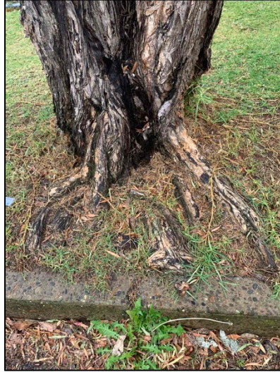
Figure 2: Surface roots of Tree 1 damaging gutter.
