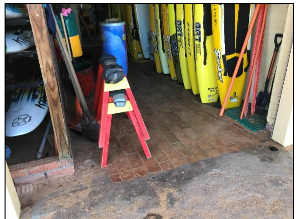
Figure 85. Detail of floor in storage area behind roll-up shutter doors. (Source: Heritage 21, 23.05.18)
