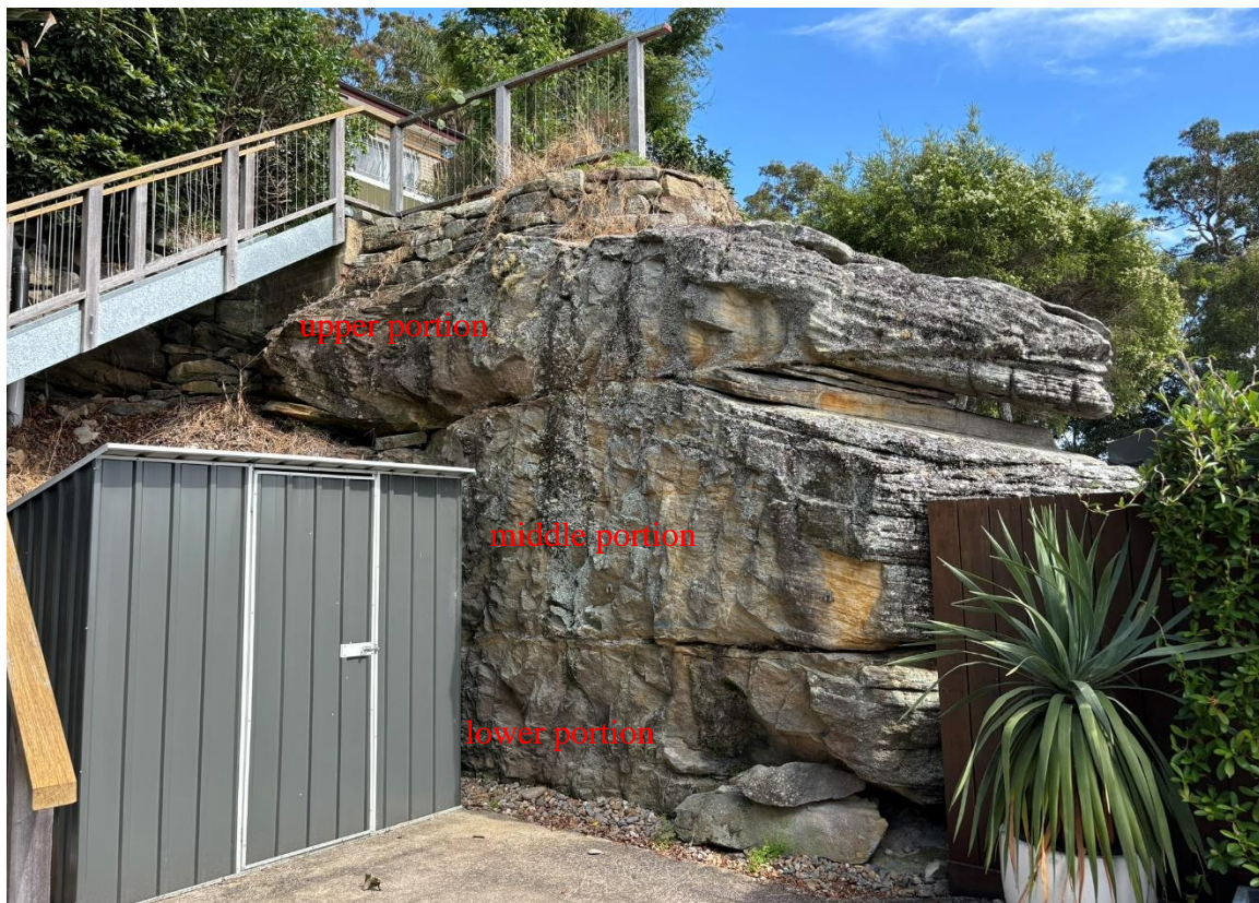
Photograph 1: View of the sandstone bedrock outcrop adjacent to the site parking space, facing northwest
