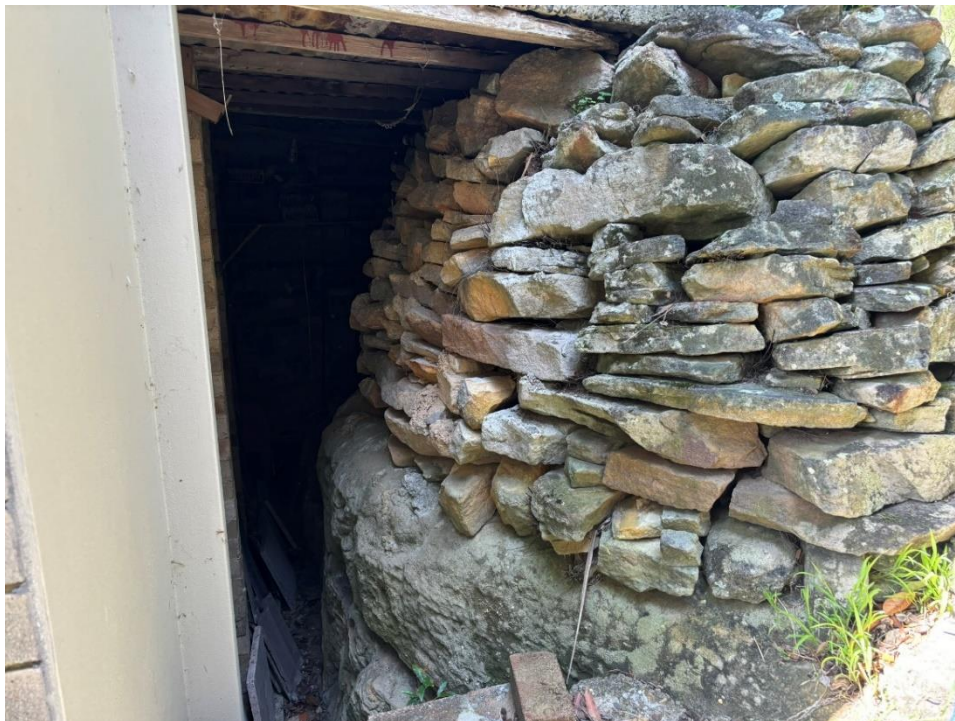
Photograph 2: View of the exposed sandstone bedrock and overlying retaining wall adjacent to the rear wall of the main structure, facing south
