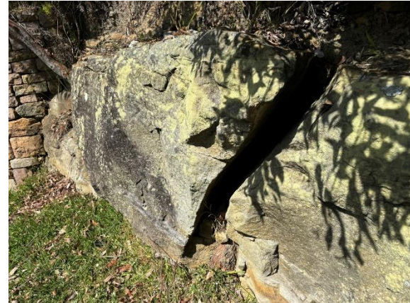
Photograph 4: Joint within exposed bedrock at the rear of the site facing southwest
