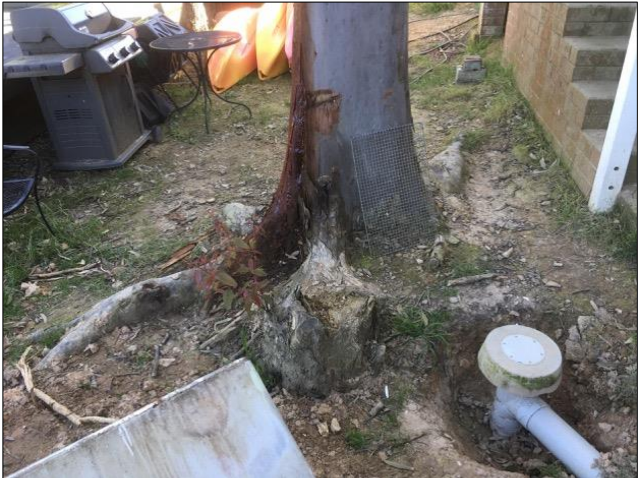
Figure 3. Hand excavation to uncover plumbing has exposed structural roots within heavy clay soil.
