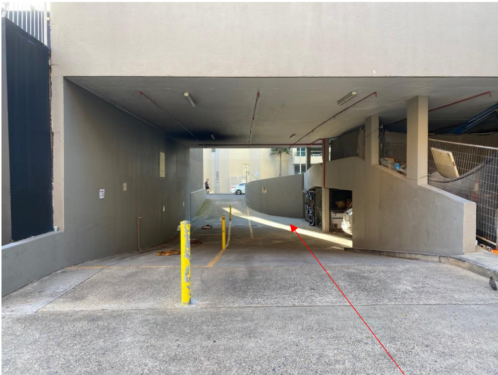
Photograph of the loading area from Short Street – area to be enclosed with new door and roller shutter
