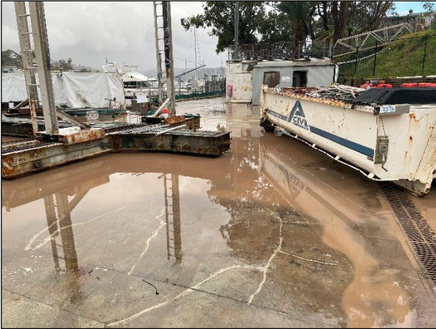
Figure 1 – Stagnant Water on the concrete hardstand
