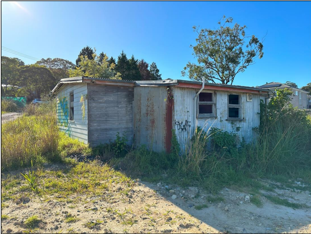
Site Photograph 6.2.2 Shed located within the north-western portion of 45 Warriewood Road, as observed on 21 June 2023.
