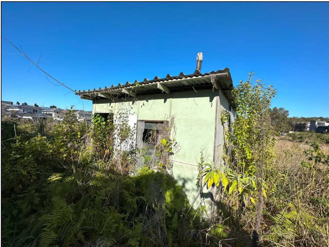
Site Photograph 6.2.5 Fibre cement structure located within the north-western portion of 45 Warriewood Road, as observed on 21 June 2023.
