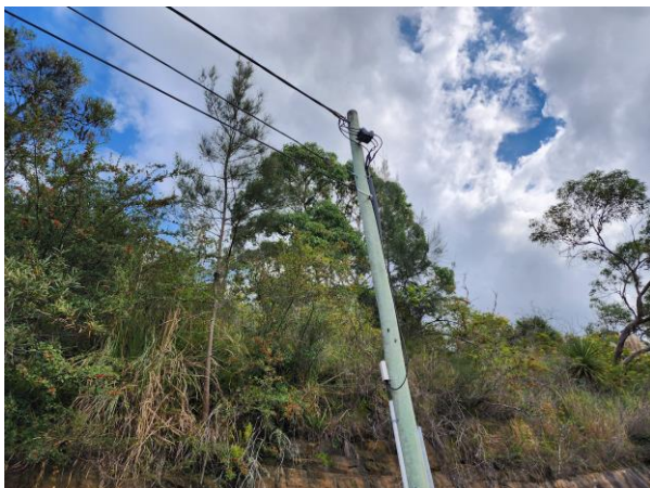
Above ground electrical supply redirection point
