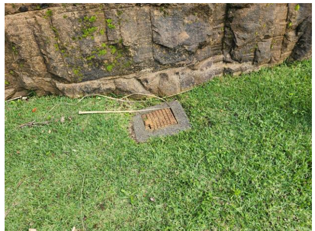
Reticulated water hydrant in pathway
