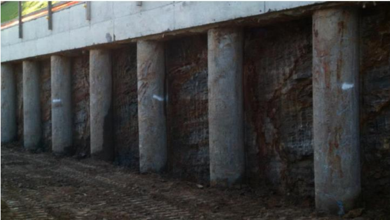
Plate 1: Photograph of Soldier Pile Wall Prior to being Shotcreted (Figure 3 from Witt Report)
