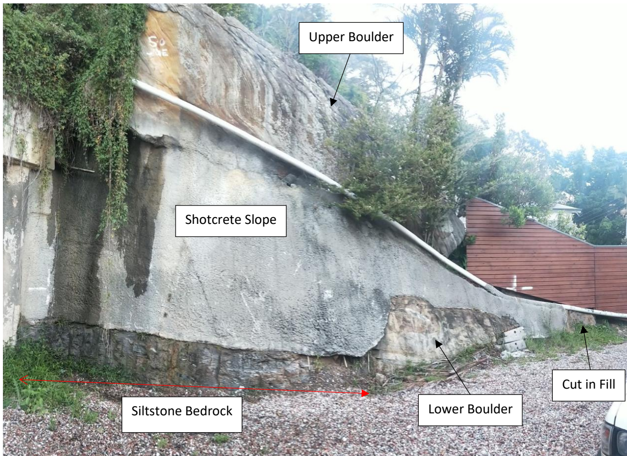
Plate 2: Photograph 1 of Large Boulders and Shotcreted Cut Face At/Near Southern Boundary (Facing South)
