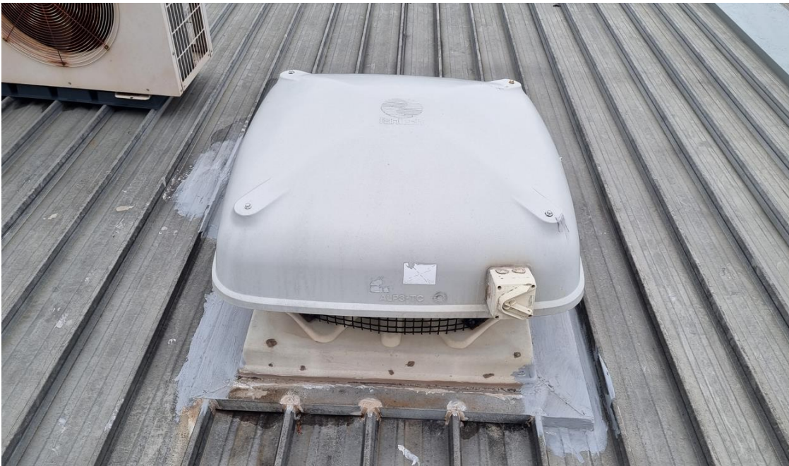
Image 5.2 – Western fan (assumed to be a fresh air intake)
