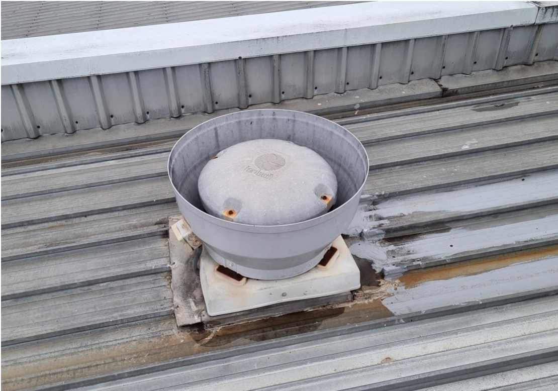
Image 5.1 – Eastern fan (assumed to be bathroom exhaust)
