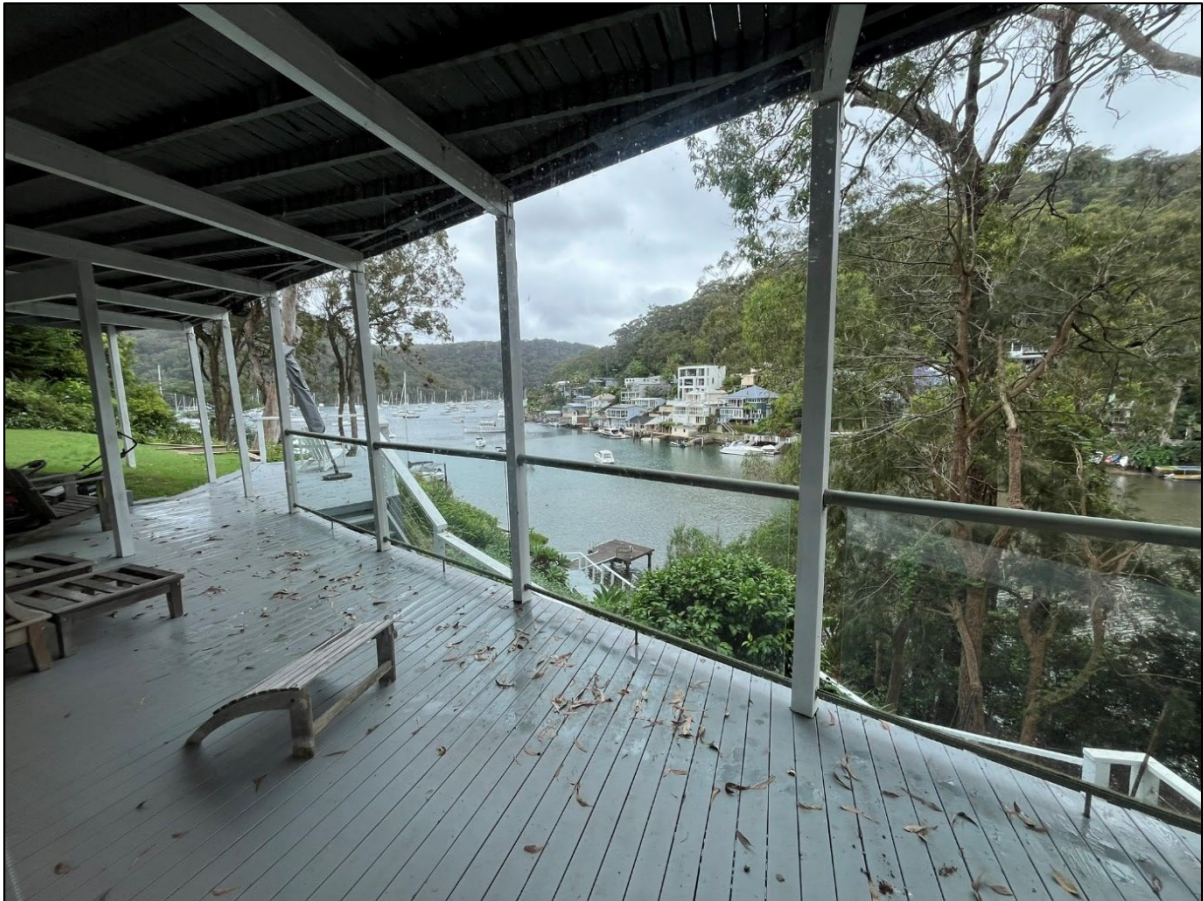
Photo 7: View to the west across the existing lower ground level deck which sits beneath the ground level deck above (see Photo 6).
