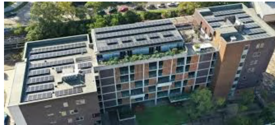
Typical apartment building PV panel installation
