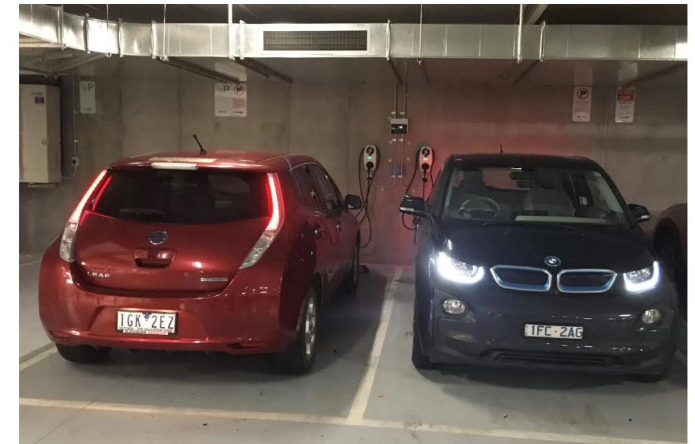
Example of EV charging provision image from https://evse.com.au/blog/apartmentevcharger/
