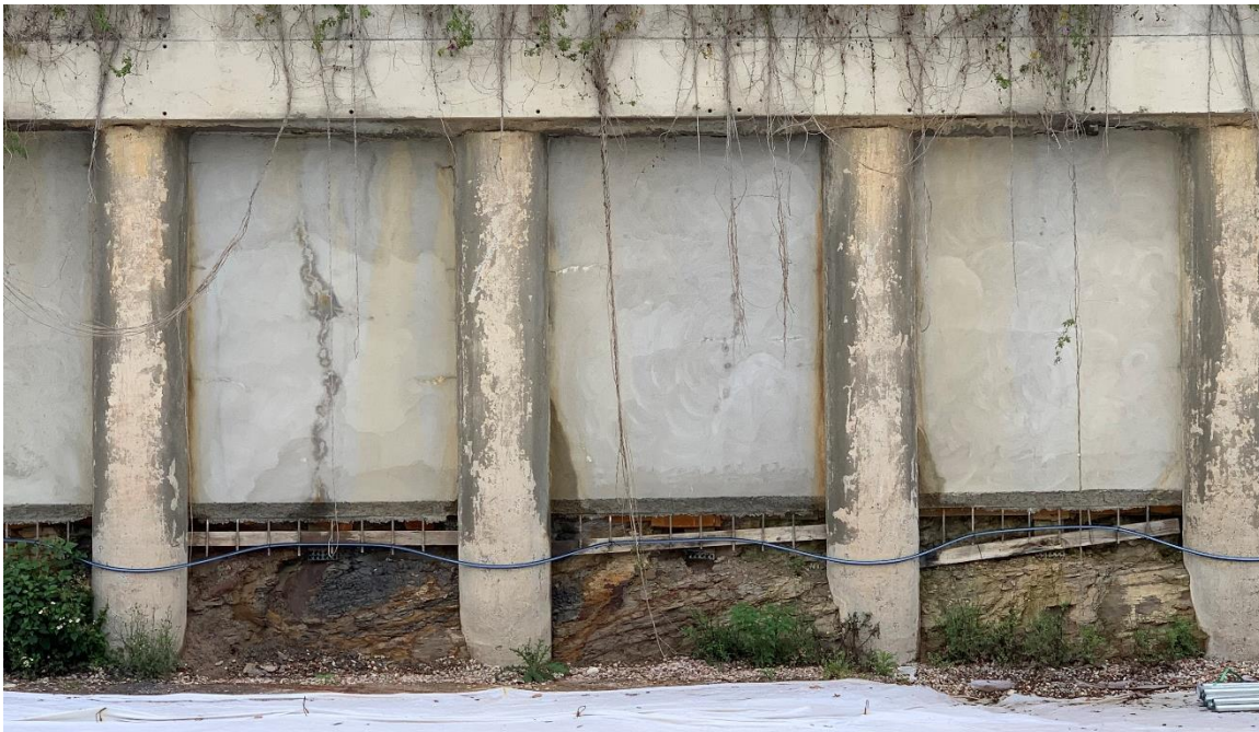
Photograph-11: Exposed siltstone and shale bedrock at the base of the concrete panel soldier pile wall at the rear excavation face of No.1104 Barrenjoey Road.
