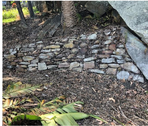
Photograph-4: Retaining wall to the north of sandstone boulder along the eastern edge of the middle-terraced region, looking east
