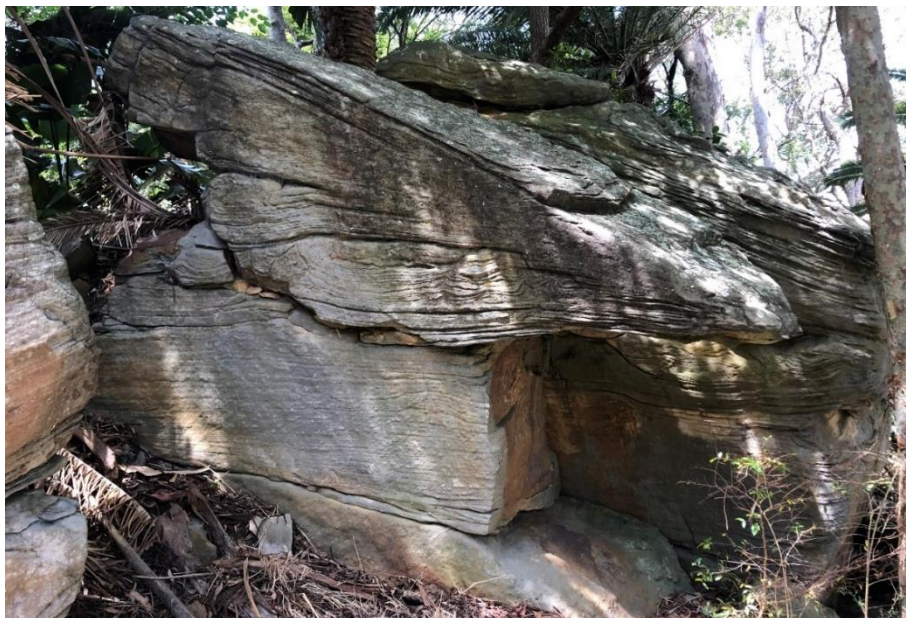
Photograph-6: Southern view of boulder instability region, including the upper triangle boulder bearing onto the lower rectangular boulder and embedded boulder below.
