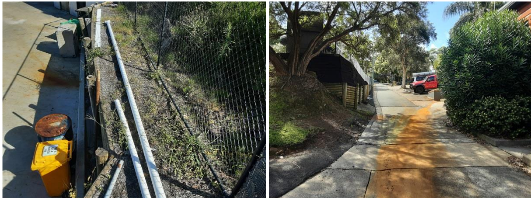
Figures 3-4 and 3-5 showing iron oxide discolouration identified onsite
