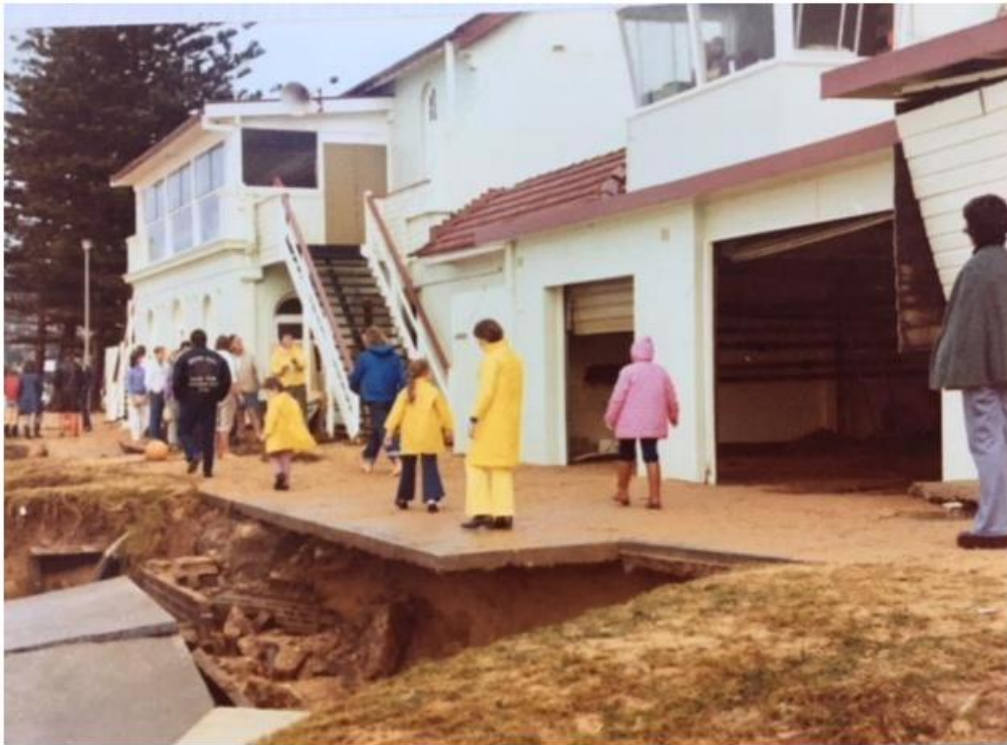
Figure 10. The Club Building in 1974 following a storm, Source: (Jennings 2009)
