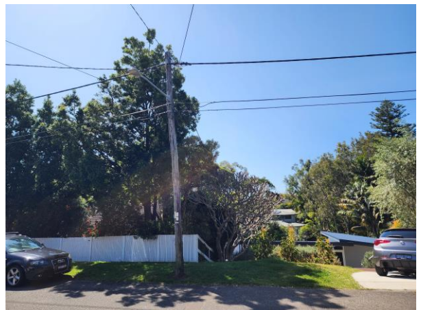
Existing electrical supply
