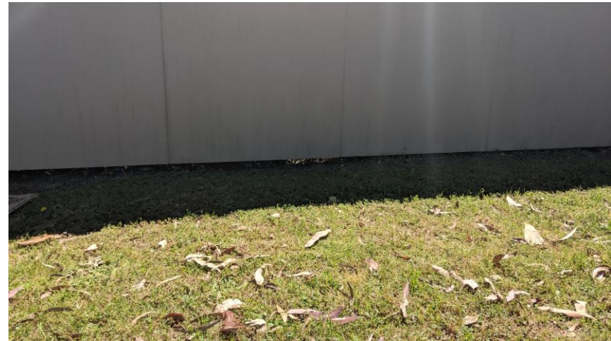
Image 2 - Gaps below existing wall (South Creek Rd)
