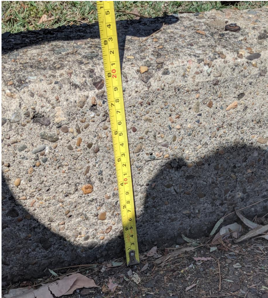
Image 1 - Kerb height, South Creek Road (south alignment)
