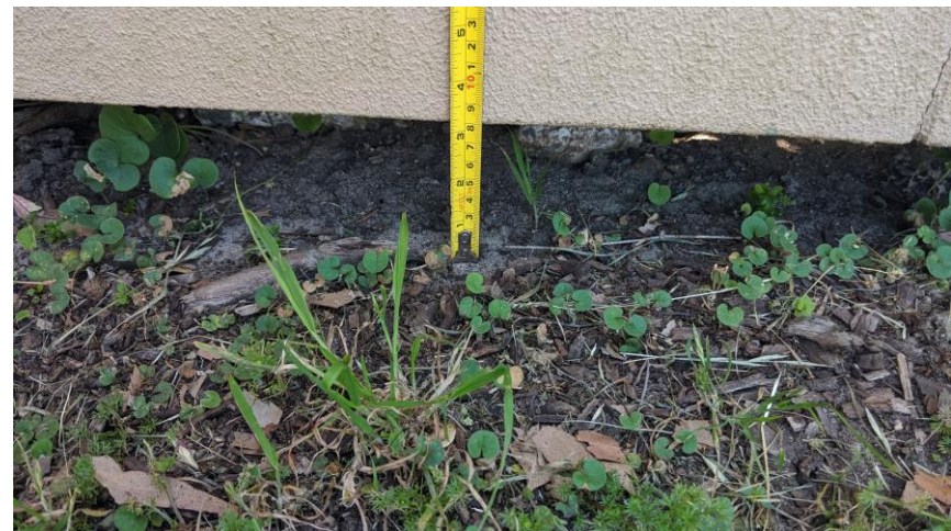
Image 3 - Gap below existing wall (South Creek Rd)
