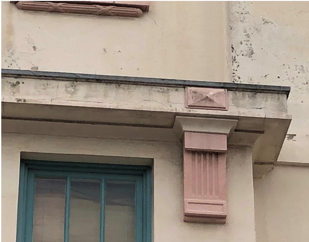
Figure 20: Detail of entablature over the first floor central bay and detailing below window sills at each level
