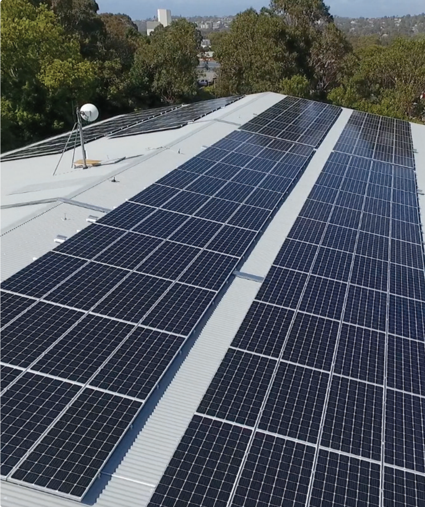
Solar panel on Council's Cromer office building roof
