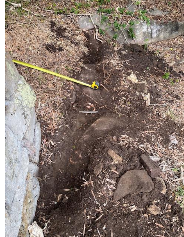
Figure 3: Root investigation trench
