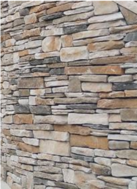
Stone walls in existing driveway/garage and also for basement + ground floor walls
