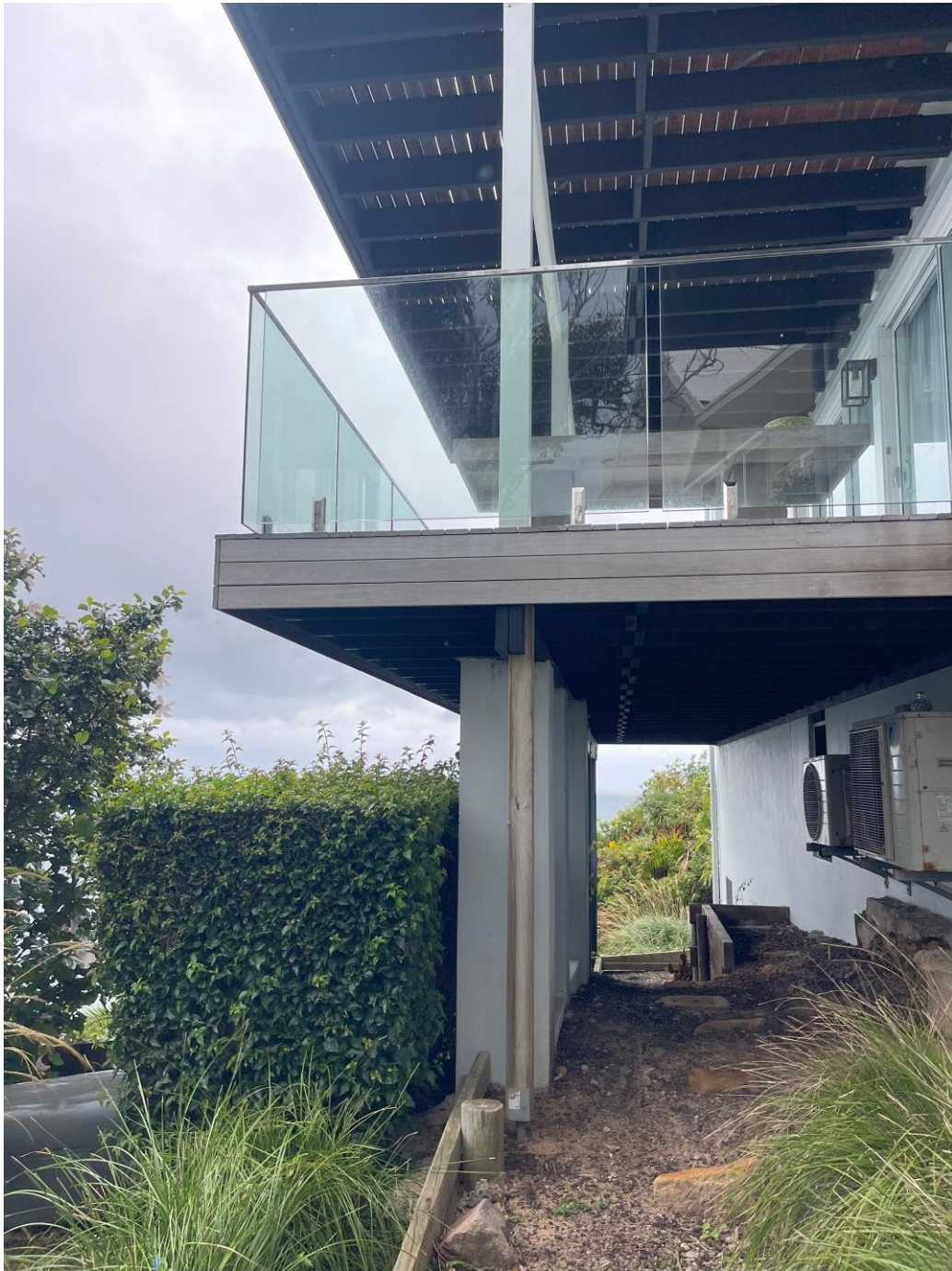
Fig 4: View of the existing undercroft area to the rear elevated decks, looking south-east
