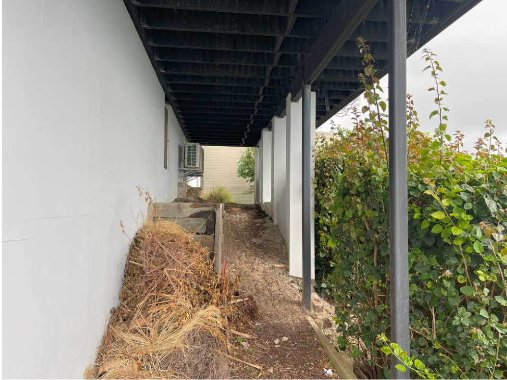
Fig 5: View of the existing undercroft area to the rear elevated decks, looking north-west
