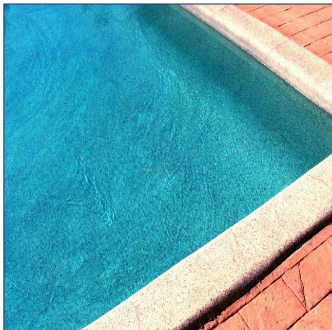
A leaking pool can waste thousands of litres of water.
