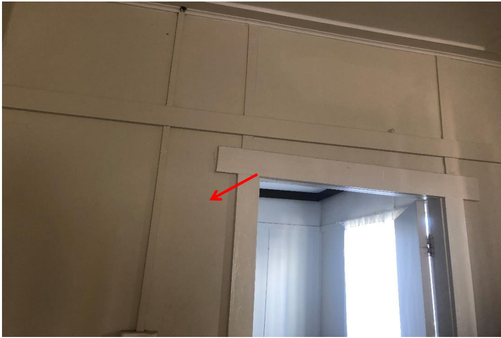
Photograph 25: 2 Dee Why Parade, Dee Why, internal, level 2, apartment 2, SE bedroom, north wall, fibre cement sheeting, asbestos detected by analysis.
