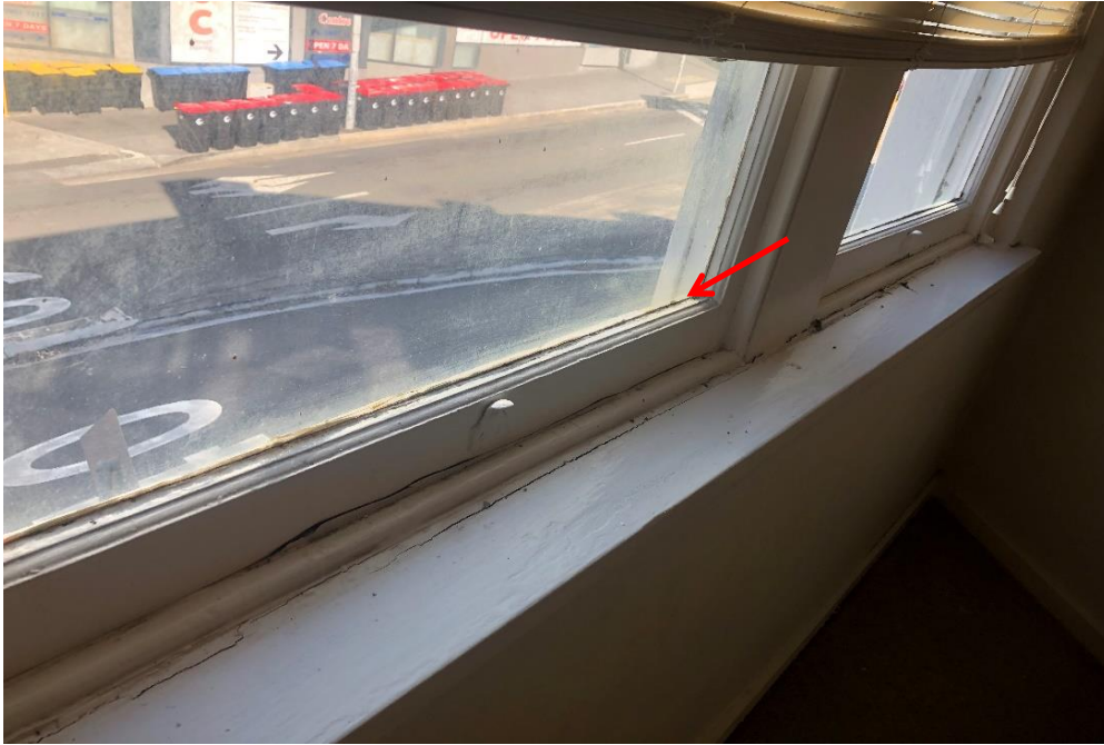
Photograph 27: 2 Dee Why Parade, Dee Why, internal, level 2, apartment 1 and 2, window mastic to non-sliding windows, bituminous material, no asbestos detected by analysis.
