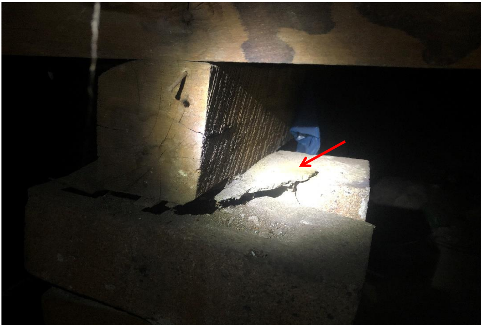
Photograph 12: 2 Dee Why Parade, Dee Why, external, subfloor areas, packing material, fibre cement sheeting, asbestos detected by analysis.
