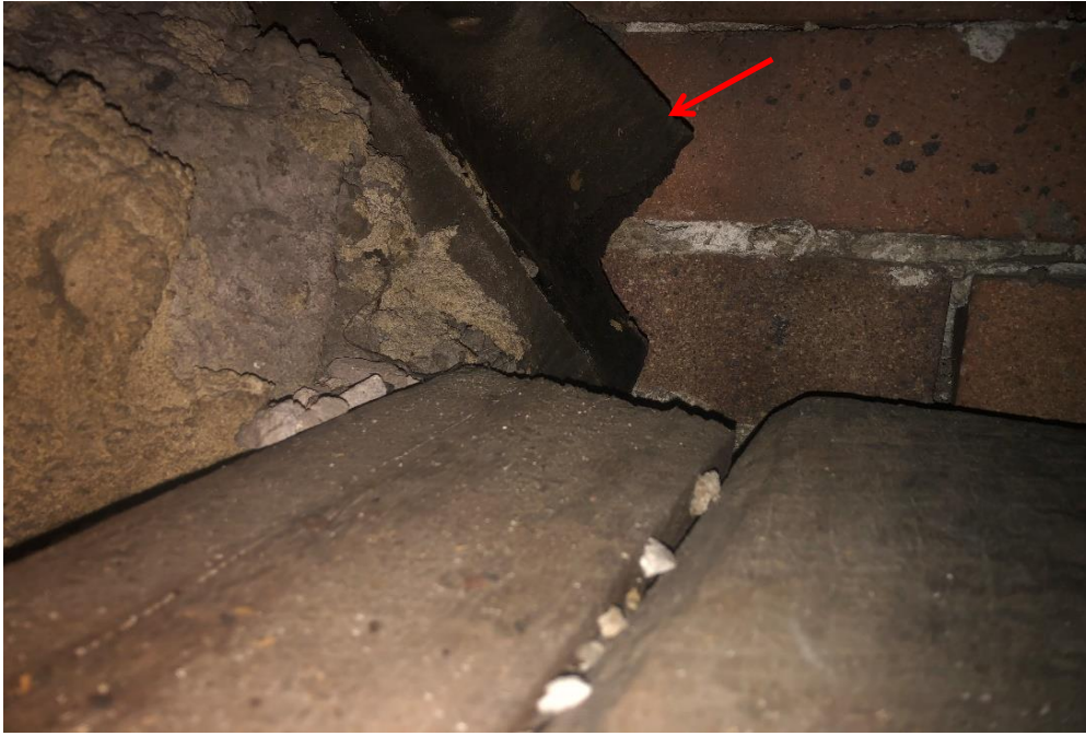
Photograph 31: 2 Dee Why Parade, Dee Why, internal, ground floor, mezzanine area, SW corner, bituminous material, no asbestos detected by analysis.
