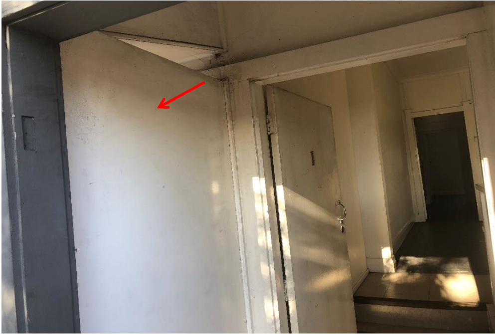
Photograph 17: 2 Dee Why Parade, Dee Why, external, level 2, adjacent apartment front doors, partition and walls, paint covering, typical gloss cream paint, non-lead paint ( \leq 0.1\% lead w/w)
