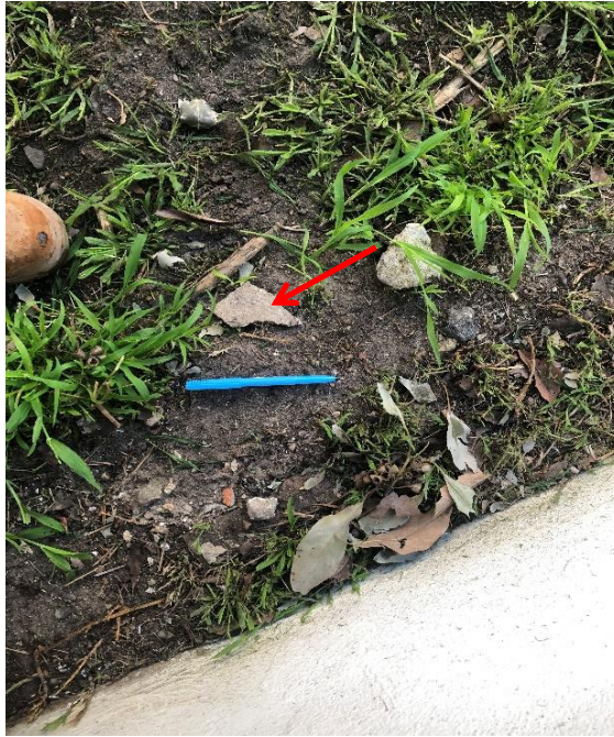
Photograph 3: 2 Dee Why Parade, Dee Why, external, south east corner, ground debris, fibre cement sheeting, asbestos detected by analysis.
