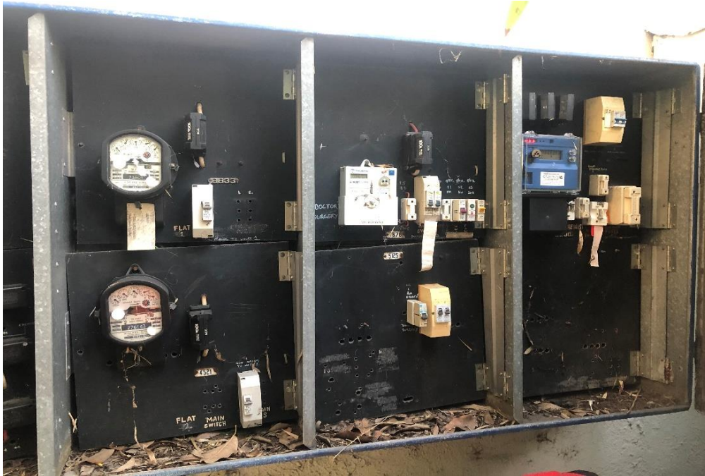
Photograph 1: 2 Dee Why Parade, Dee Why, external, southeast corner, electrical box, electrical backing board(s), suspected asbestos.
