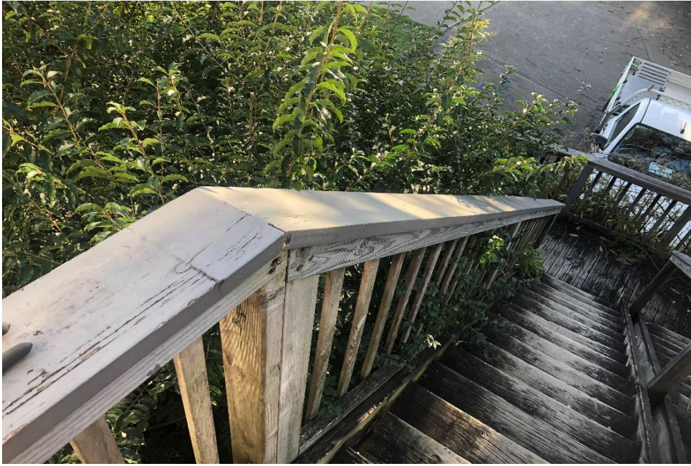
Photograph 15: 2 Dee Why Parade, Dee Why, external, north elevation, stair handrail to level 2, paint covering, typical grey paint, non-lead paint ( \leq 0.1\% lead w/w)
