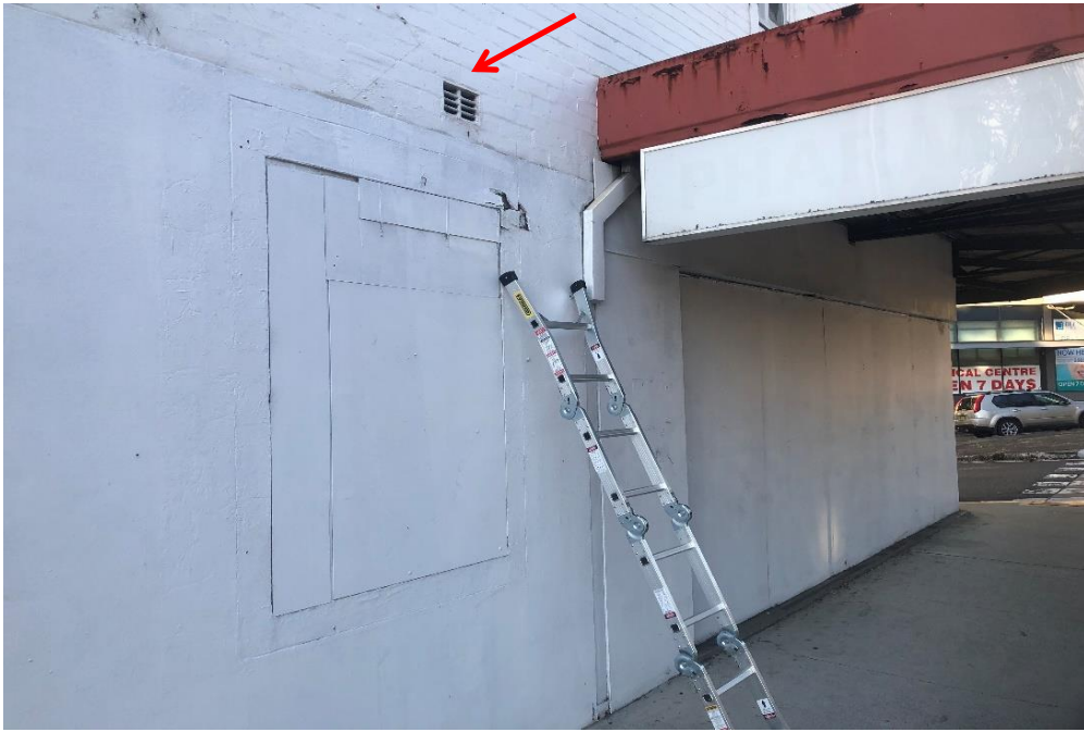
Photograph 7: 2 Dee Why Parade, Dee Why, external, surfaces throughout, paint covering, typical off-white paint, non-lead paint ( \leq 0.1\% lead w/w)
