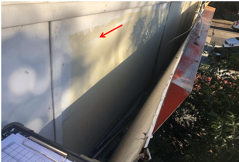
Photograph 18: 2 Dee Why Parade, Dee Why, external, walls throughout, undercoat paint covering, typical cream paint, non-lead paint ( \leq 0.1\% lead w/w)
