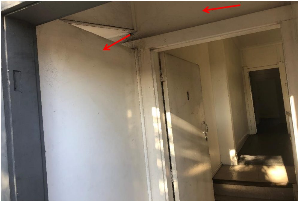
Photograph 16: 2 Dee Why Parade, Dee Why, external, level 2, adjacent apartment front doors, partition and walls, fibre cement sheeting, no asbestos detected by analysis.
