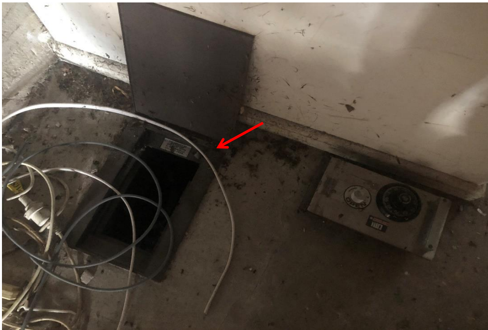
Photograph 32: 2 Dee Why Parade, Dee Why, internal, basement storage area, north elevation, in floor safe, safe lining, suspected non-asbestos.
