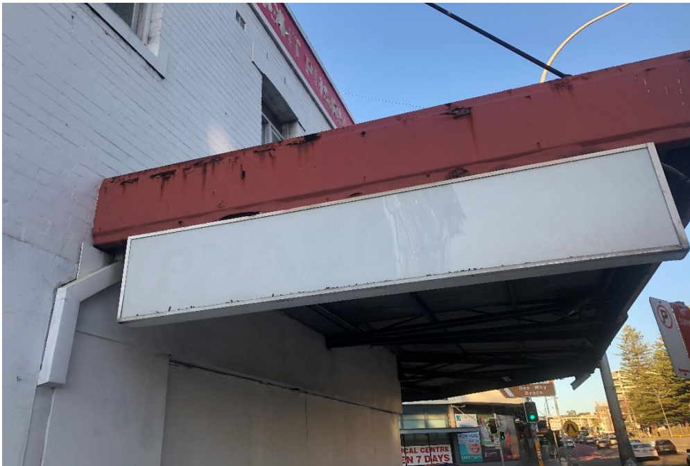
Photograph 6: 2 Dee Why Parade, Dee Why, external, surfaces throughout, paint covering, light red paint, lead paint (>0.1% lead w/w).
