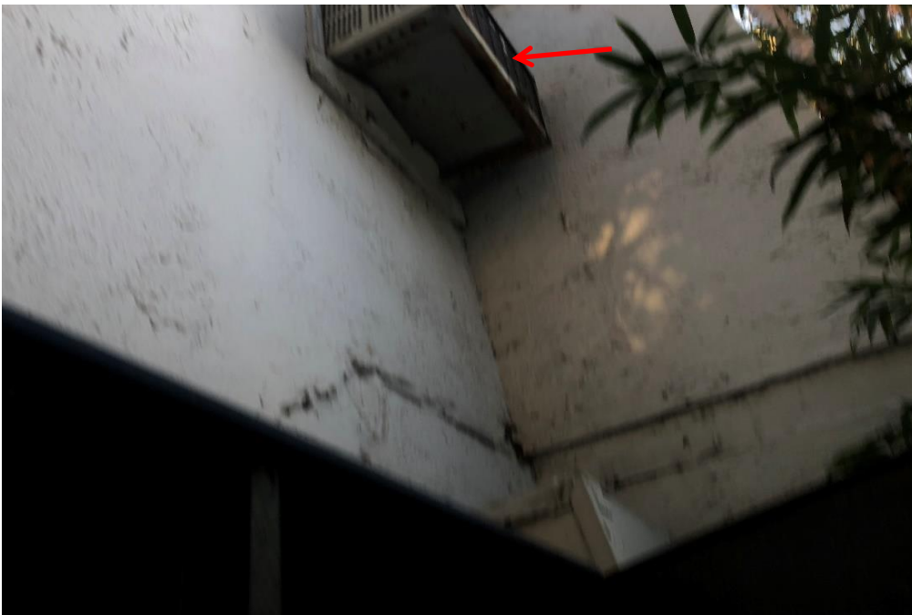
Photograph 2: 2 Dee Why Parade, Dee Why, external, southeast corner and throughout, A/C unit(s), bulk internal insulation, suspected SMF.
