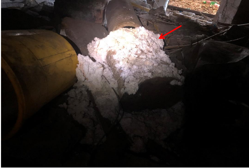
Photograph 13: 2 Dee Why Parade, Dee Why, external, subfloor areas, central subfloor area, suspect insulation material, no asbestos detected by analysis.
