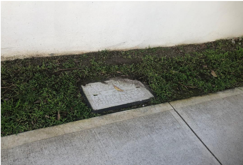
Photograph 4: 2 Dee Why Parade, Dee Why, external, southern elevation, service pit, suspected non-asbestos.
