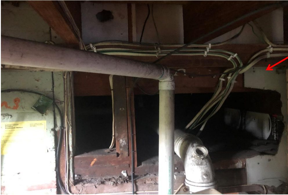
Photograph 11: 2 Dee Why Parade, Dee Why, external, subfloor areas, infill panels, throughout, fibre cement sheeting, asbestos detected by analysis.
