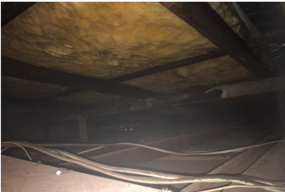
Photograph 24: 2 Dee Why Parade, Dee Why, internal, level 2, apartment 1, roof space, ceiling dust, elevated lead (10.2 mg/m2).
