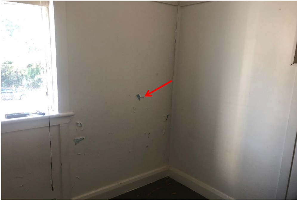
Photograph 21: 2 Dee Why Parade, Dee Why, internal, level 2, apartment 1 and 2, wall paint covering, throughout, typical white paint, non-lead paint ( \leq 0.1\% lead w/w).
