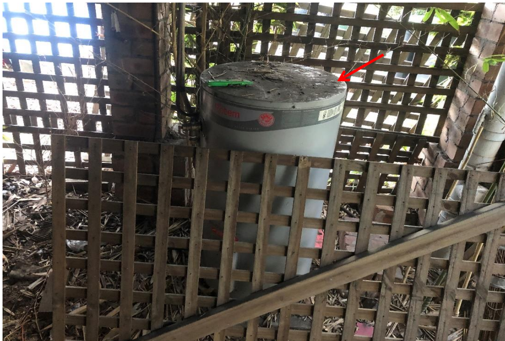
Photograph 14: 2 Dee Why Parade, Dee Why, external, subfloor areas, rheem hot water system, bulk internal insulation, suspected SMF.
