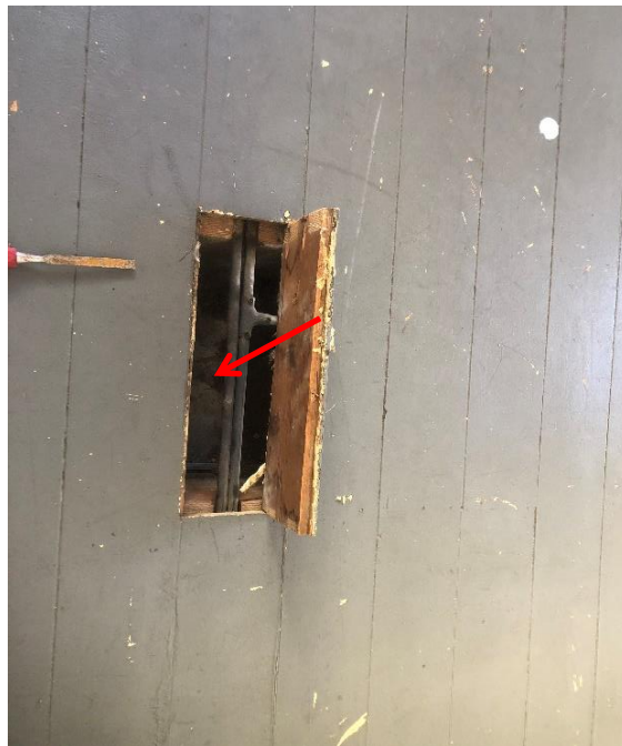
Photograph 22: 2 Dee Why Parade, Dee Why, internal, level 2, apartment 1, main bedroom, cavity below floorboards (possibly throughout), fibre cement sheeting, asbestos (assumed).
