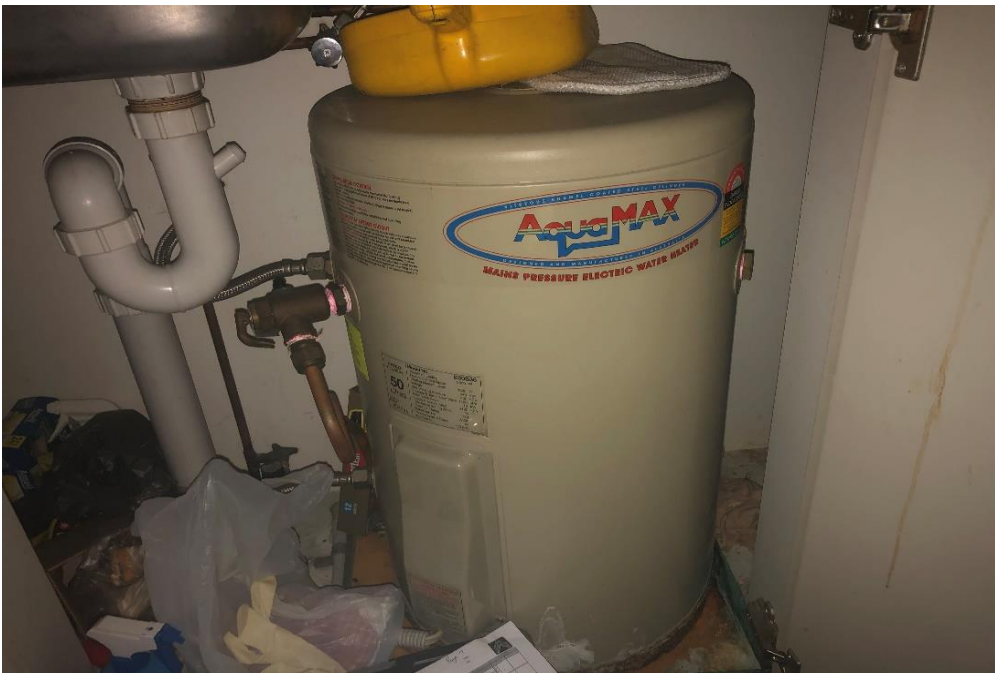
Photograph 30: 2 Dee Why Parade, Dee Why, internal, ground floor, kitchenette, aqua max hot water system, bulk internal insulation, suspected SMF.
