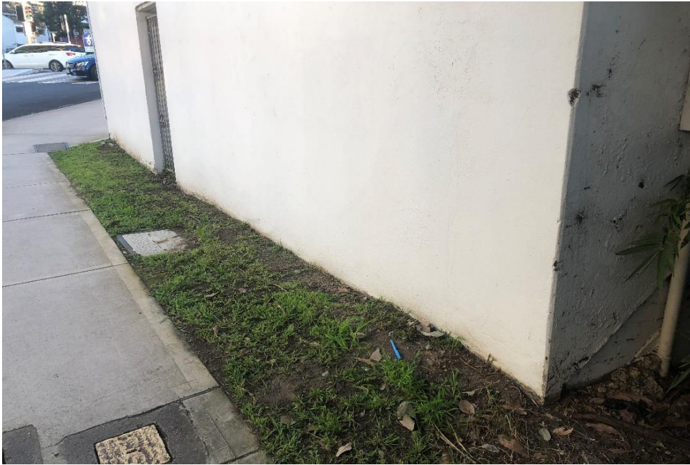
Photograph 5: 2 Dee Why Parade, Dee Why, external, surface throughout, paint covering, white paint, lead paint (>0.1% lead w/w).
