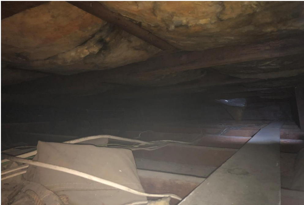
Photograph 28: 2 Dee Why Parade, Dee Why, internal, level 2, apartment 2, roof space, ceiling dust, elevated lead (77.8 mg/m 2 ).
