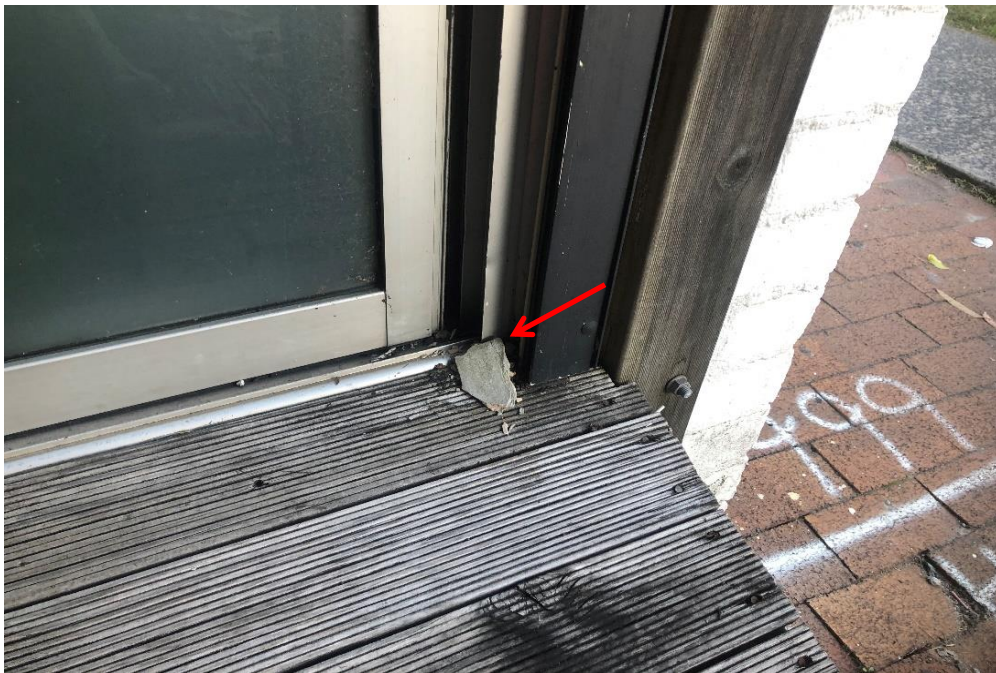
Photograph 8: 2 Dee Why Parade, Dee Why, external, western elevation, ramp to hair salon, ground debris, fibre cement sheeting, no asbestos detected by analysis.
