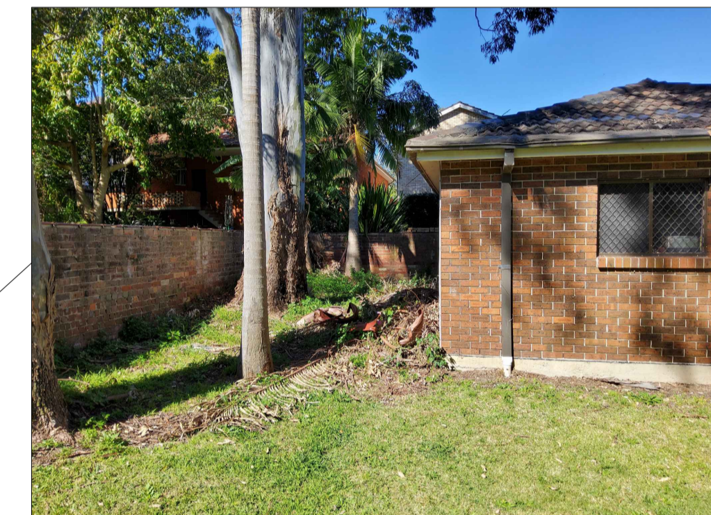
EXISTING BRICK MASONRY ALONG EASTERN BOUNDARY TO BE RETAINED AND REPAIRED FOR REUSE
