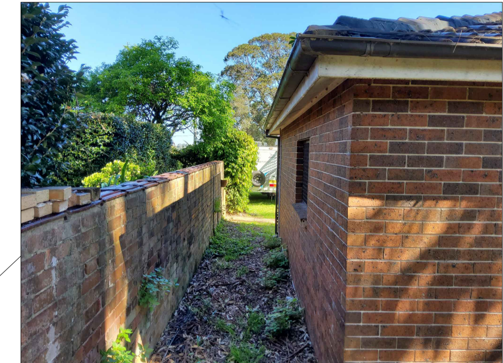
EXISTING BRICK MASONRY ALONG EASTERN BOUNDARY TO BE RETAINED AND REPAIRED FOR REUSE
